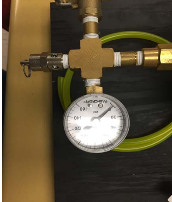
Figure 73: Safety Valve and Gage
