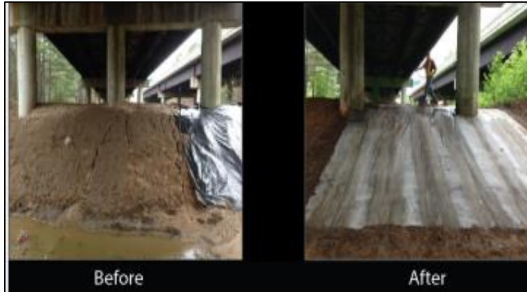
Figure 36: Example of concrete blanket effects (Milliken Infrastructure)
