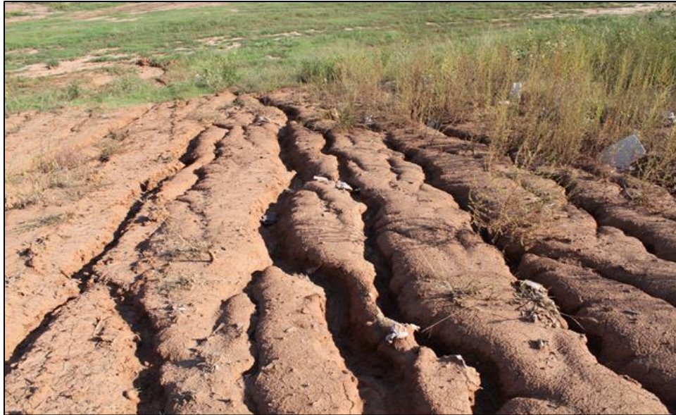
Figure 2: Image of current rill erosion issue
