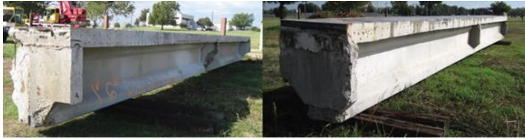
Figure 15: Two views of girder C showing details of condition on October 8, 2013
