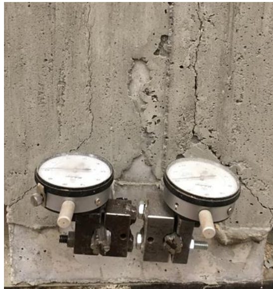
Figure 96: Diaphragm cracking at girder interface
