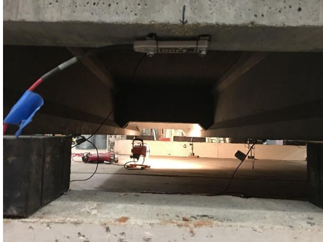
Figure 81: BDI gauge attached to center of end diaphragm
