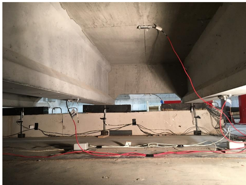
Figure 152: Scale bridge instrument locations, including strain gauge at center of slab span (top of picture)
