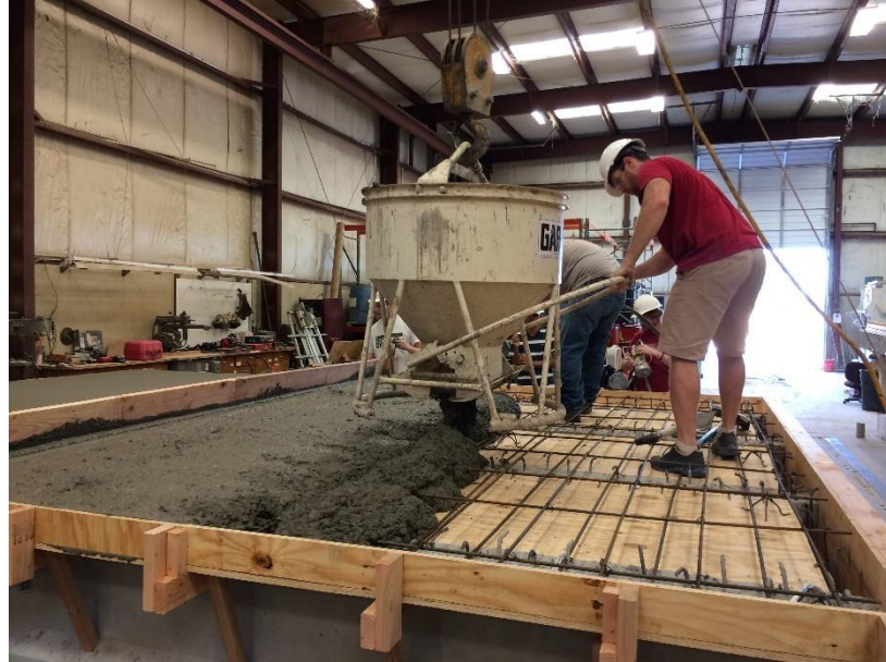
Figure 75: Discharging concrete into deck forms, screeding operation visible on left of photo
