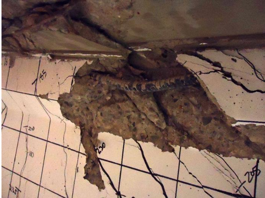
Figure 52: Buckling of compression steel in girder flange and failed deck concrete
