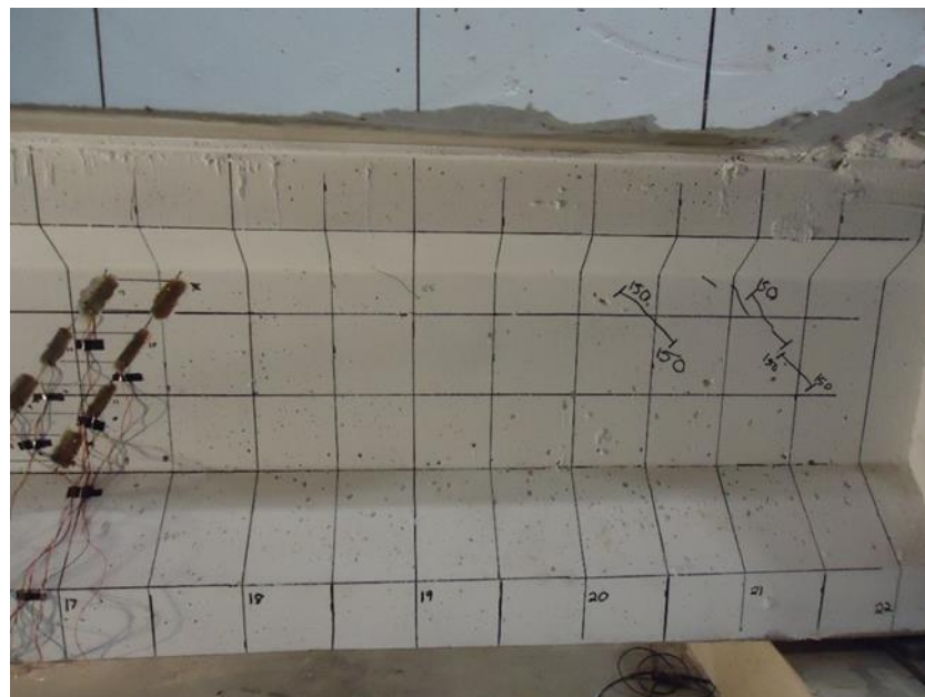
Figure 48: Initial cracking in test C2
