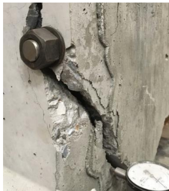
Figure 104: Failure at diaphragm connection
