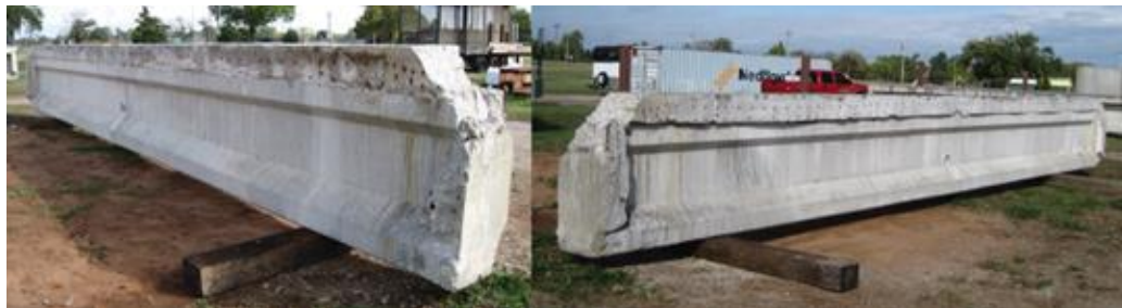
Figure 14: Two views of girder A showing details of condition on October 8, 2013
