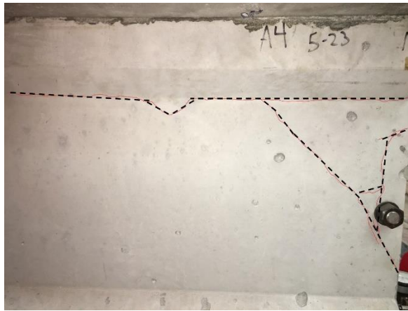
Figure 103: Cracking around diaphragm connection in the southernmost outside girder (A4)
