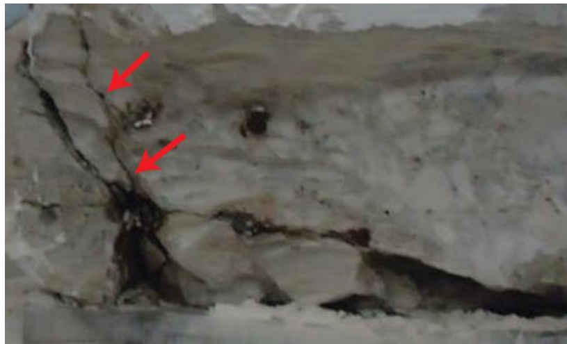
Figure 39: Spalling and cracking at girder end initiated by corrosion cracks
