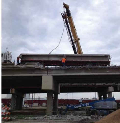
Figure 10: Removal of girder C from the I-244 bridge over the Arkansas river in Tulsa, OK on September 4, 2013 (photo courtesy of Gary Quinonez with Manhattan Road & Bridge)
