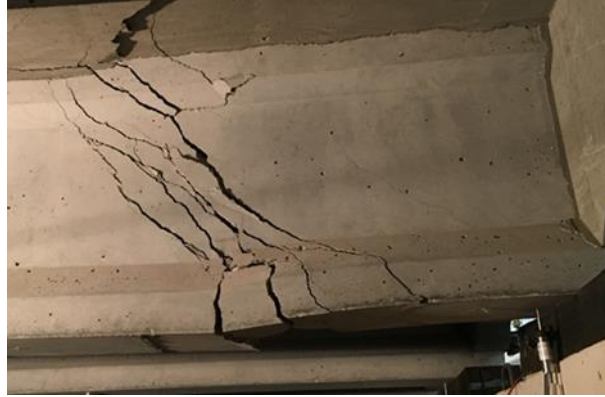
Figure 108: Final shear cracking in loaded girder, note punching in slab
