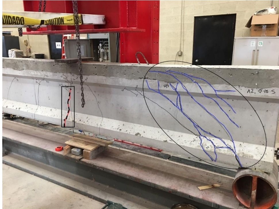
Figure 90: Cracking during test A2s, initial flexural crack (boxed) and shear cracks (circled) shown
