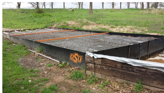
Phosphorus drainage filter installed at a poultry farm.
