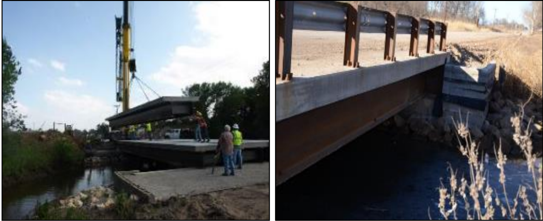
Figure 73: Bridge No. 5 - GRS-IBS with concrete block facing (geotextile reinforcement needs to be trimmed)
