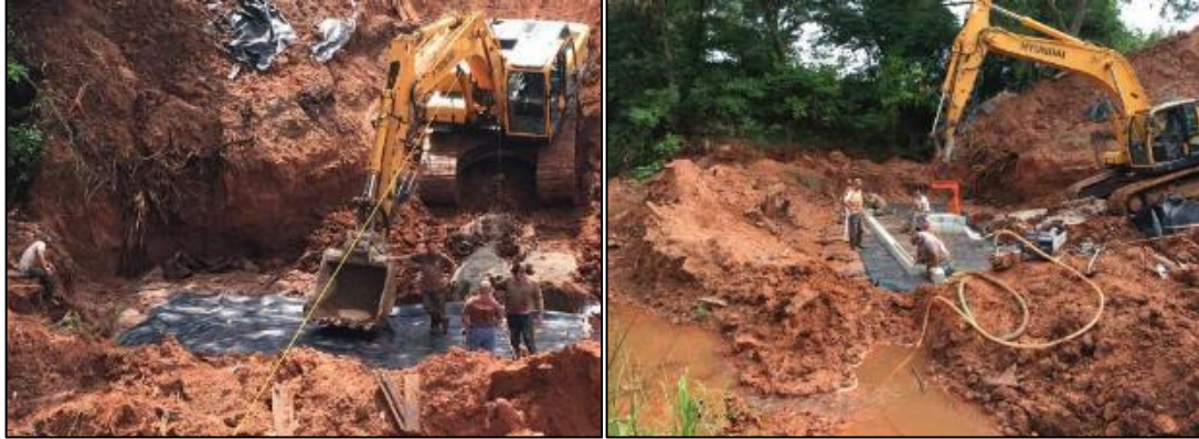
Figure 53: Pumping of flood water out of the GRS abutment site, and placement of a new reinforcement layer on the top of the RSF
