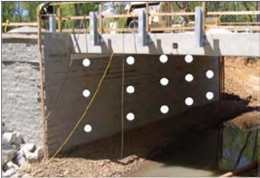
Figure 27: Survey points on the abutment of 1-366 Bridge in Delaware (Talebi et al.2014)
