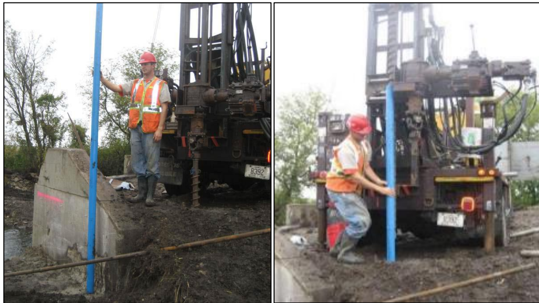
Figure 25: Three 5-foot inclinometer casings snapped together during installation on a bridge abutment in Delaware (Vennapusa 2012)
