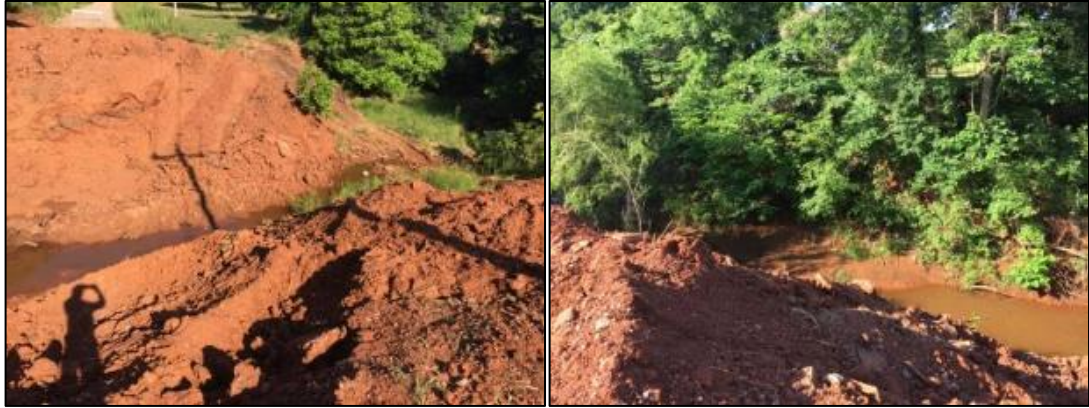
Figure 51: Yates Bridge site after demolition of old bridge and excavation for new GRS abutments
