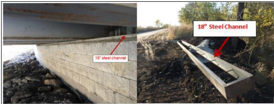
Figure 71: Bridge No. 2 - GRS-IBS with an 18 in.-wide concrete-filled steel channel as the bearing pad for the steel girders
