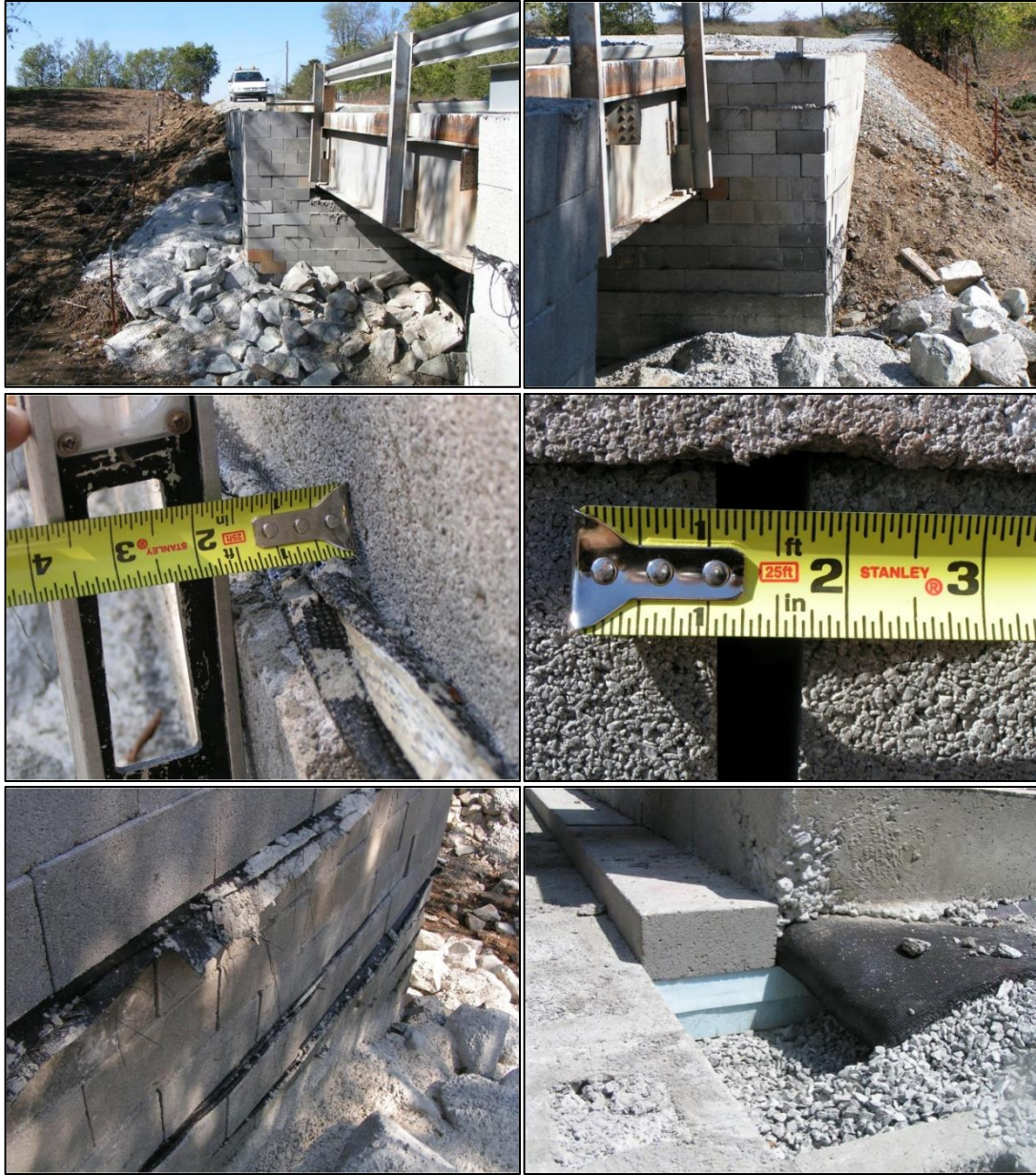
Figure 48: Issues observed in the first GRS-IBS bridge in Ottawa County, OK, including leaning wing walls, gaps in facing blocks and exposed geotextile reinforcement. (Photographs courtesy of C. Westlund, PE)
