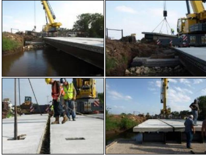
Figure 76: Different stages of GRS-IBS construction near Blackwell in Kay County, OK (photographs courtesy of Mr. Tom Simpson, PE)
