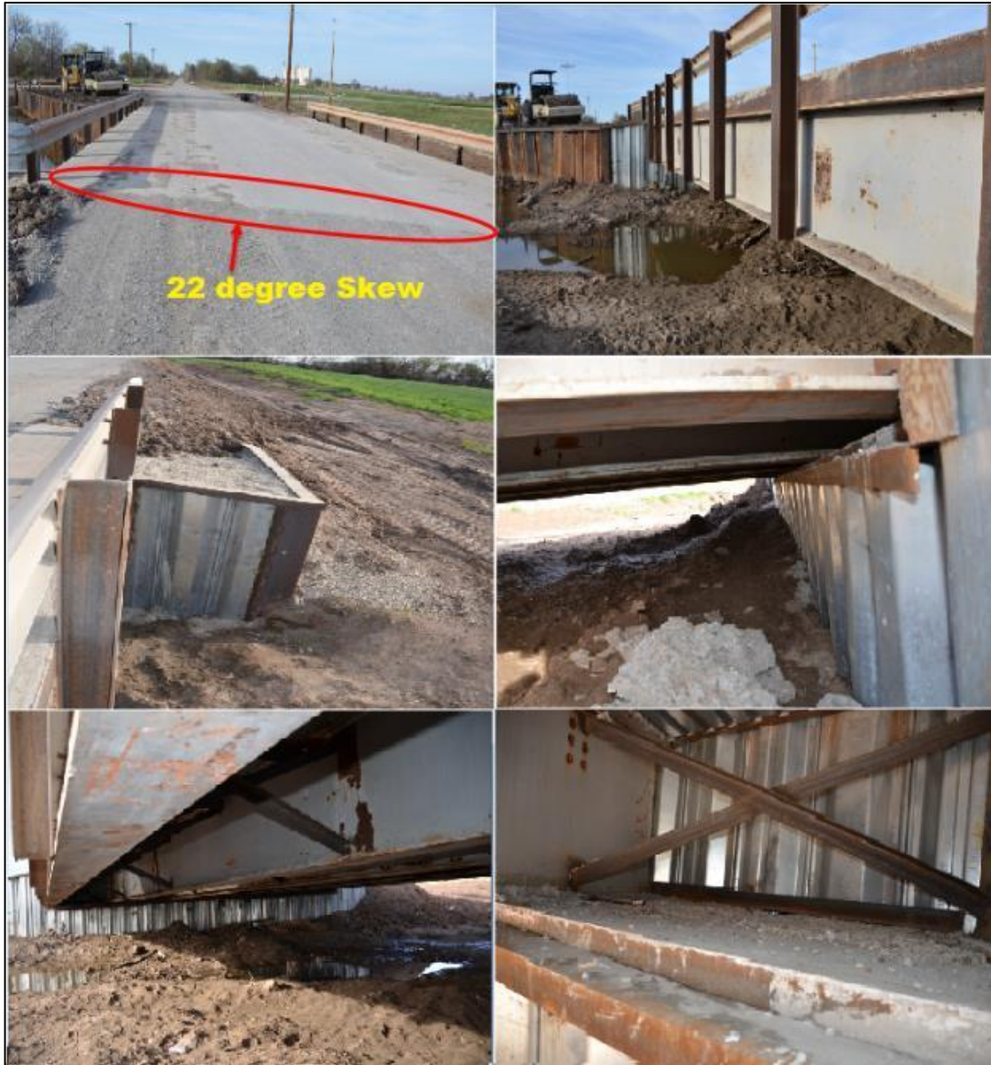
Figure 77: Completed Bridge No. 3 (GRS-IBS) with sheet pile facing (red circle indicates a 22 skew in the alignment of the bridge superstructure)
