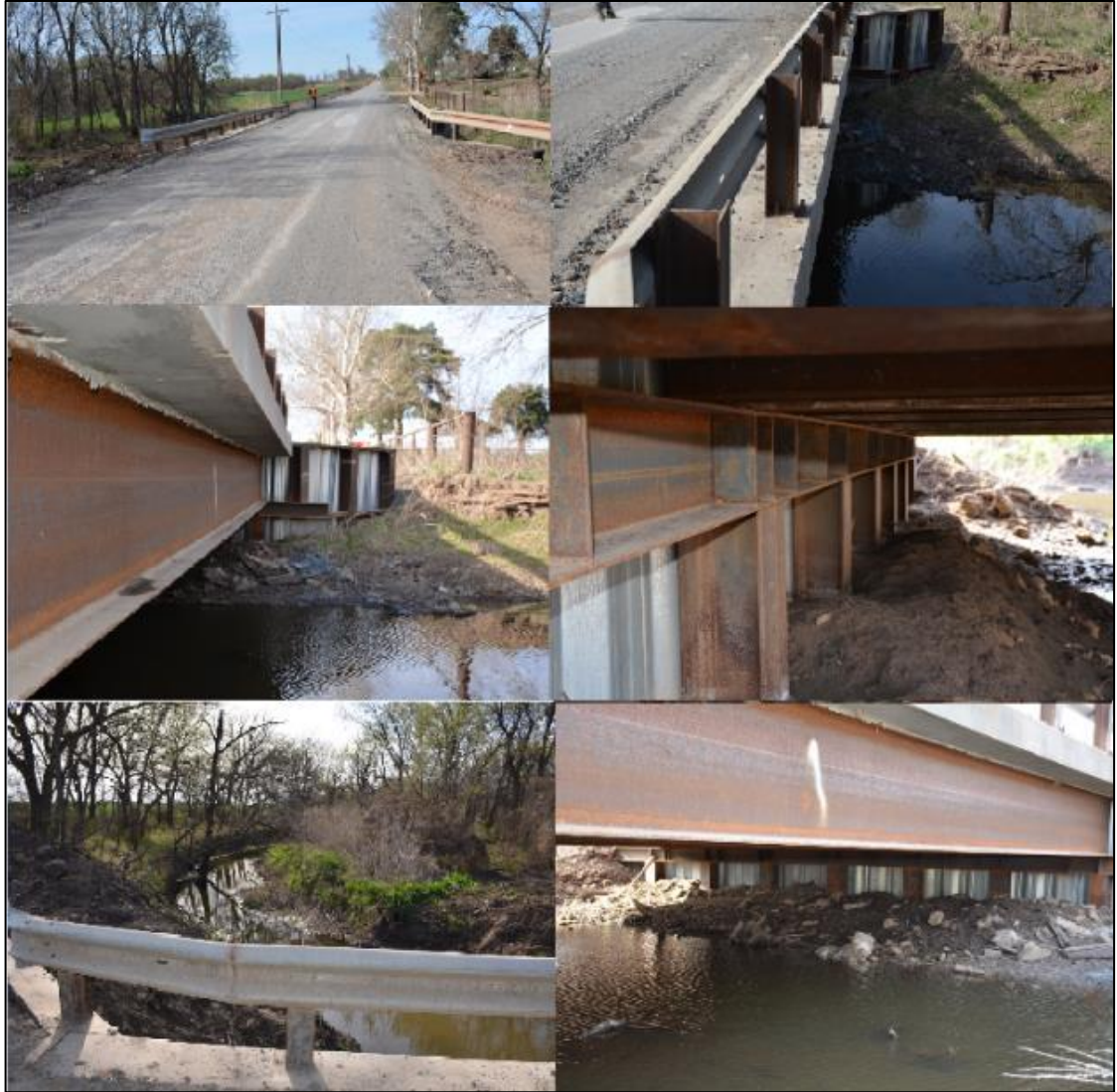
Figure 80: Completed Bridge No. 6 (conventional abutments on H-Piles driven to bedrock but with sheet pile abutment facing)
