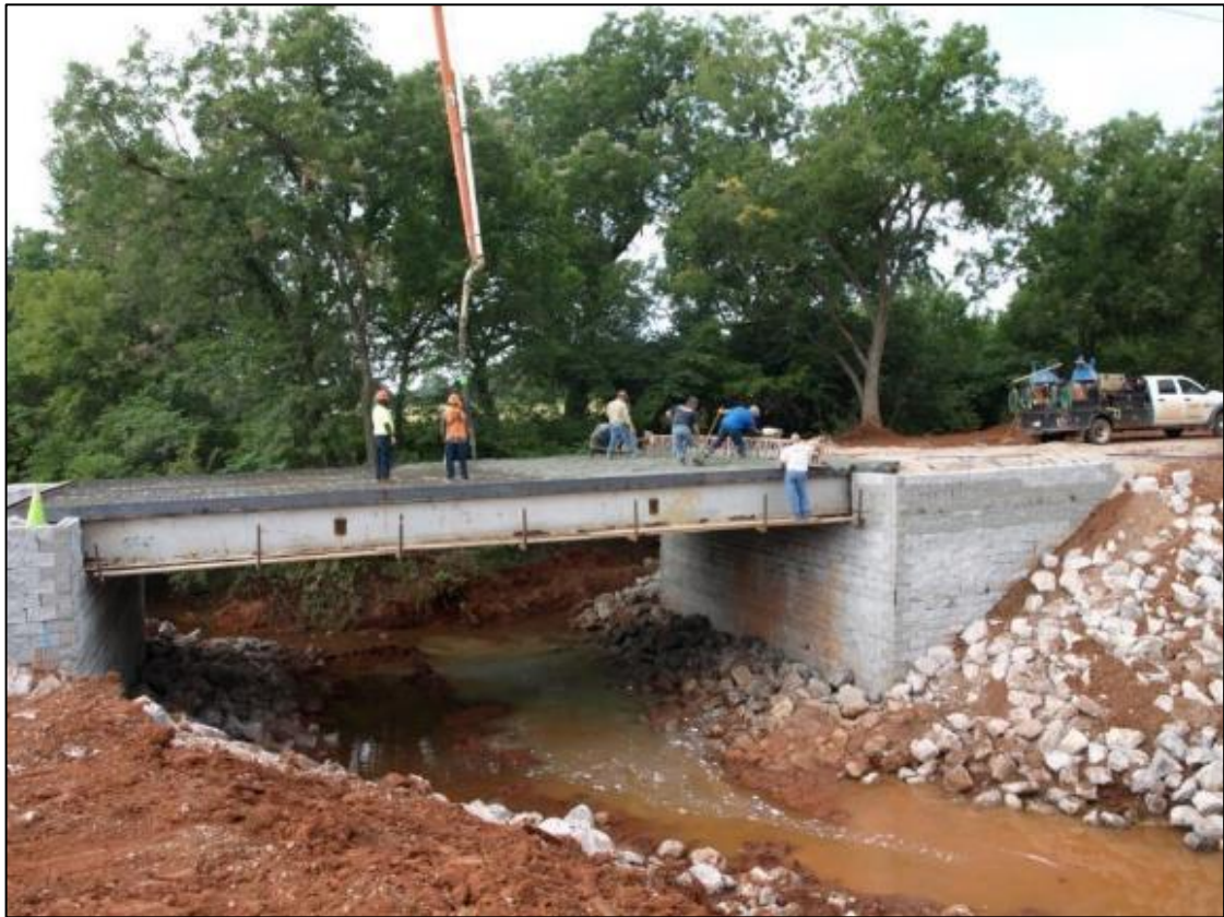
Figure 54: Construction of concrete deck at Yates Bridge, Lincoln County, OK (Photograph courtesy of Mr. Tom Simpson, PE)
