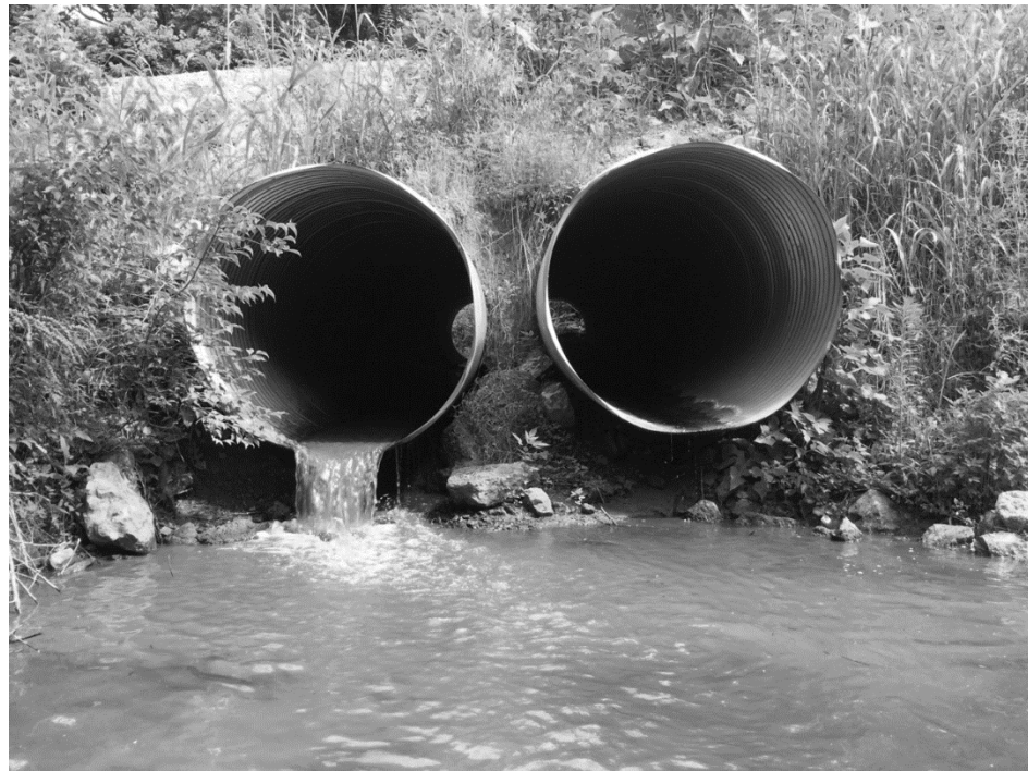
Figure 1. Image a. depicts a box culvert with a significant outlet drop, while image b. shows a round culvert with a significant outlet drop. Both of these barriers are impassable to aquatic life.
