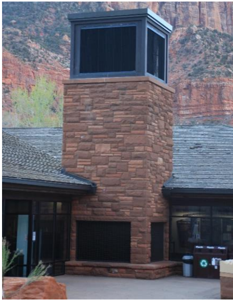
a) Wind Tower
