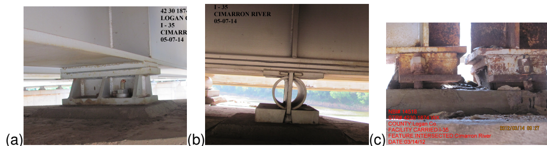
Figure 4.5: Photos of bearings used in the I-35 bridge over the Cimarron River: (a) fixed high-type steel bearing; (b) roller bearing; (c) expansion elastomeric bearing.
