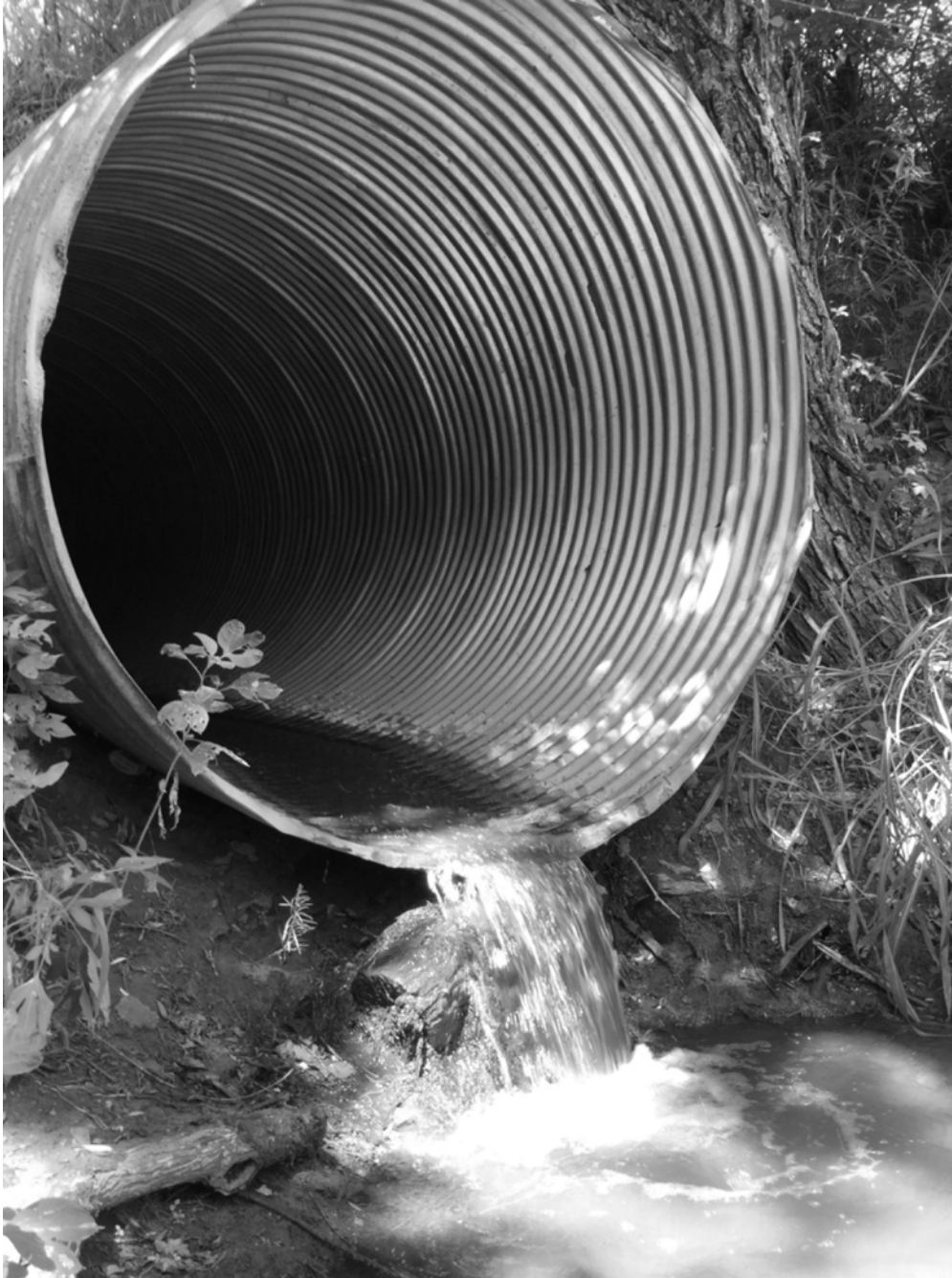
Figure 2.1: Road culverts can block the upstream movement of fishes. The presence of an outlet drop (shown here) and increased water velocity are the two most common means by which road culverts block fish movement (Janchowski-Hartley et al. 2014). Photo credit: N. Sleight.
