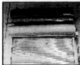
Figure 5. Air curtain installed above a roll-up dock door.
