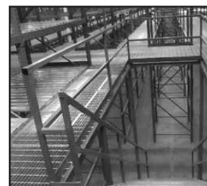
Figure 2. Overhead catwalks must not allow particles to fall through into processing areas, also, adequate kick guards should be included to prevent particles from being kicked into adjacent processing areas.
