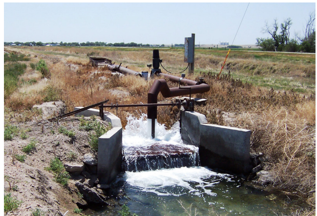
Figure 3. An electric pump discharges groundwater into an irrigation ditch.
