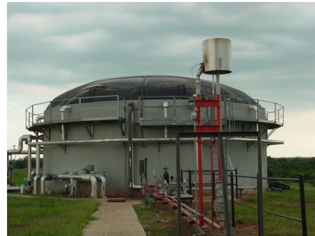
Figure 12. ASBR digester located on the Oklahoma State University Swine Research and Education Center.
