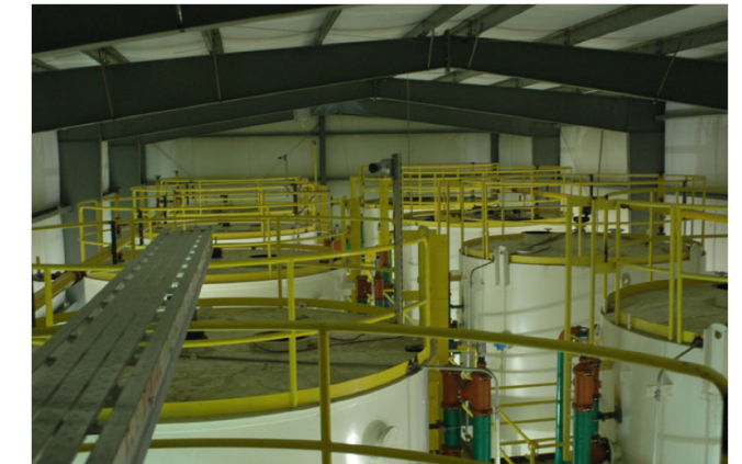
Figure 10. Battery of IBR digesters (Photo courtesy of Conly Hansen, Utah State University).
