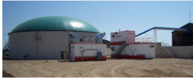
Figure 3. Complete mix digester located on the Cave Brothers Farm in Waterloo, Wis. (Photo courtesy of Cave Brothers Farm/USEPA).
