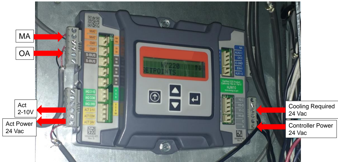
Figure 11: Photo of the economizer controller (standard commercially available JADE model controller) used in the RTU for the tests of the present work
