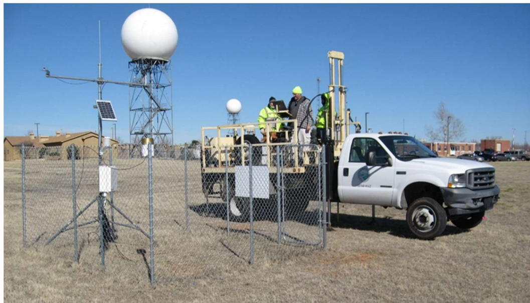
Figure 3.2: Weather station installed at North Base test site, Oklahoma Department of Transportation truck in background performing CPT.
