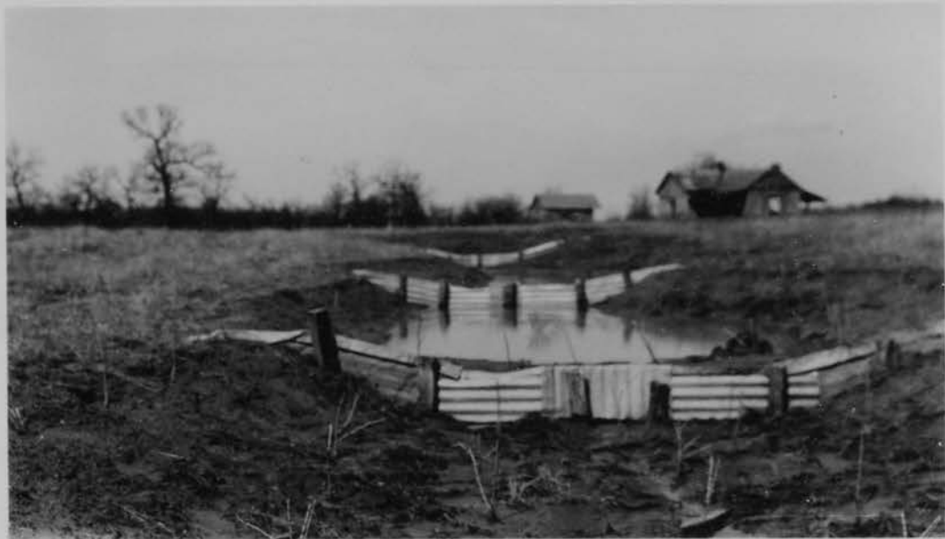
Picture No. 38 Check dams made of scrap sheet iron across a large gully. Note: The small trees growing in the foreground.
