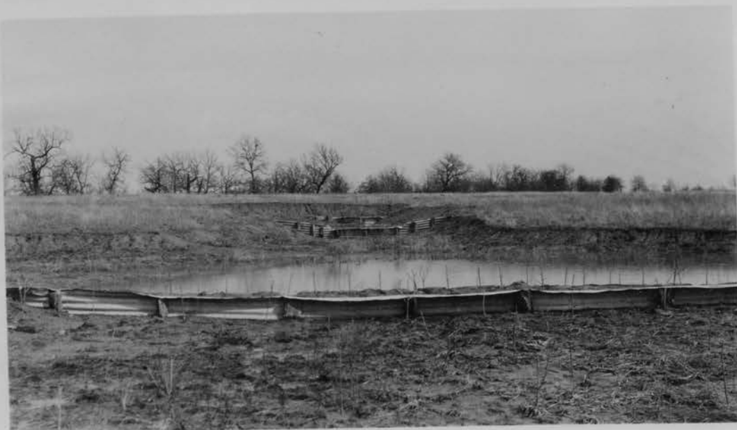
Picture No. 40 Check dams across a gully in a field which was formerly cultivated. Note: The seedling trees which were planted among the dams.
