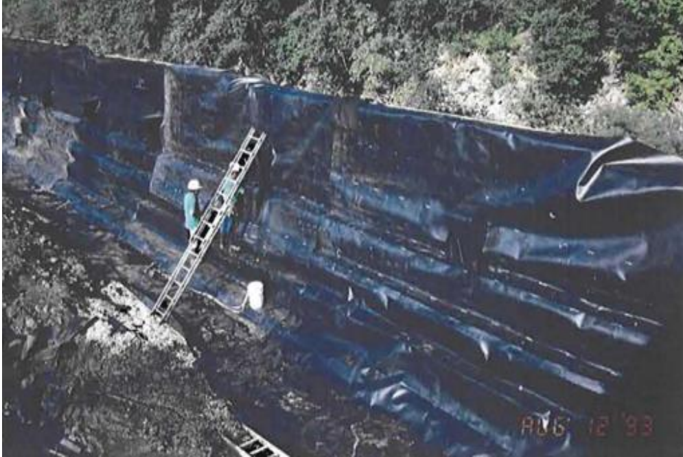
Figure 3. Image of the latest retaining wall during the installation of the groundwater extraction and treatment system from the 1990s (Gentry et al., 2013).
