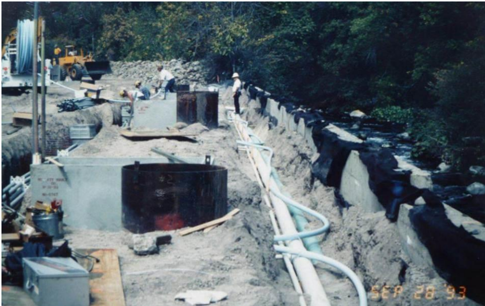
Figure 4. Image of groundwater extraction and treatment system during installation during the 1990s (Gentry et al., 2013).
