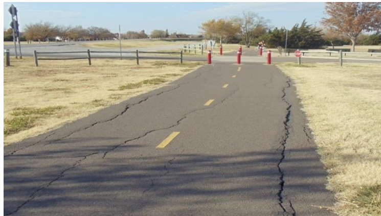
Figure 1.3 Cracks at Lake Hefner Site in Oklahoma City (Bulut et al. 2014)
