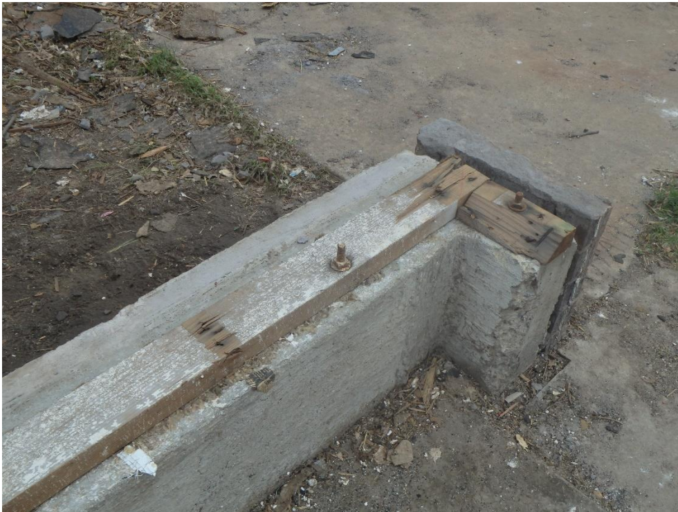
Figure 1-22 Broken Sill Plate Along the Edge (Tornado Damage Assessment in the aftermath of the May 20th 2013 Moore Oklahoma Tornado, 2014)
