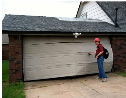
Figure 1-8 Light Grage Door Failure (Tornado Damage Assessment in the aftermath of the May 20th 2013 Moore Oklahoma Tornado, 2014)
