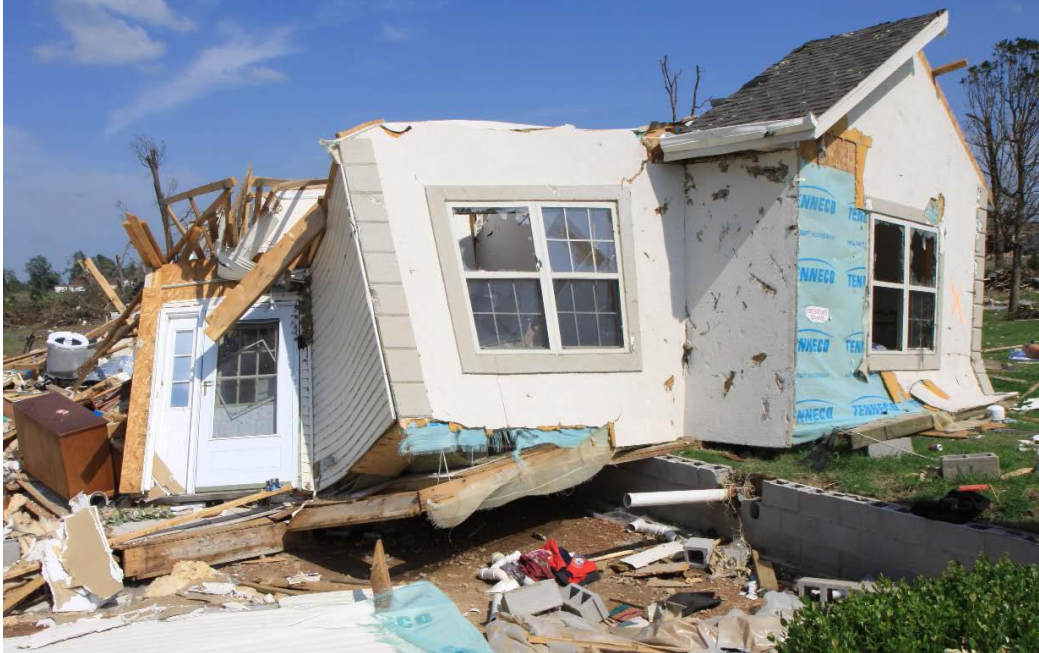
Figure 1-18 House shifted off of foundation in Joplin, MO after 2011 Tornado. (Tornado Damage Assessment in the aftermath of the May 20th 2013 Moore Oklahoma Tornado, 2014)
