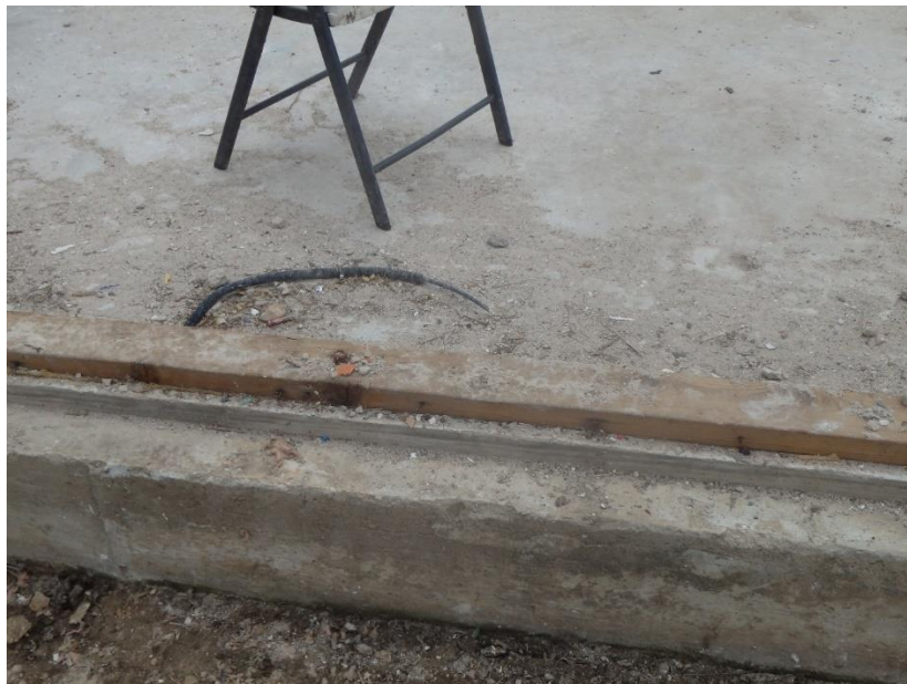
Figure 1-20 Undamaged Sill Plate (Tornado Damage Assessment in the aftermath of the May 20th 2013 Moore Oklahoma Tornado, 2014)
