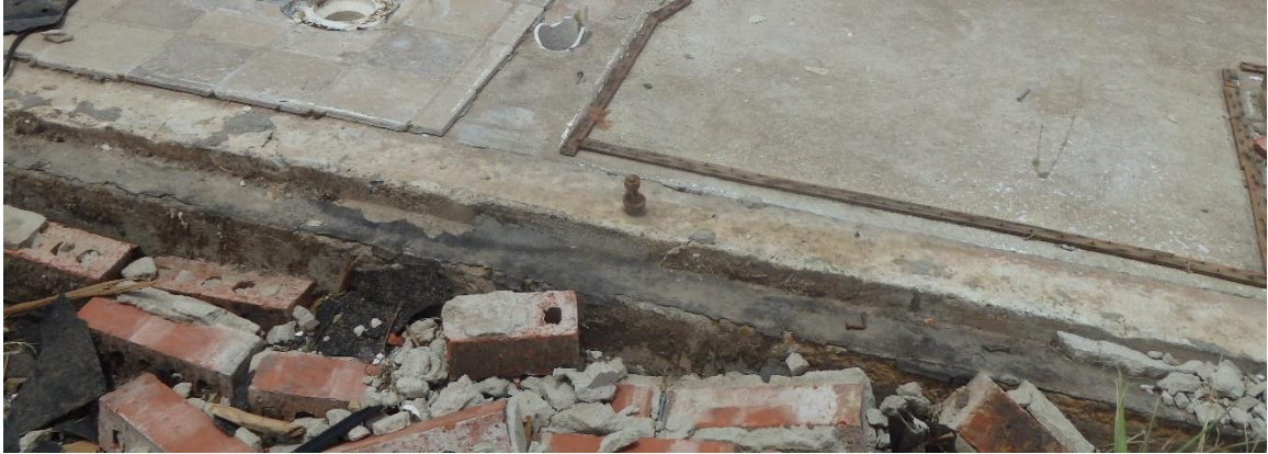
Figure 1-21 Damaged Sill Plate (Tornado Damage Assessment in the aftermath of the May 20th 2013 Moore Oklahoma Tornado, 2014)
