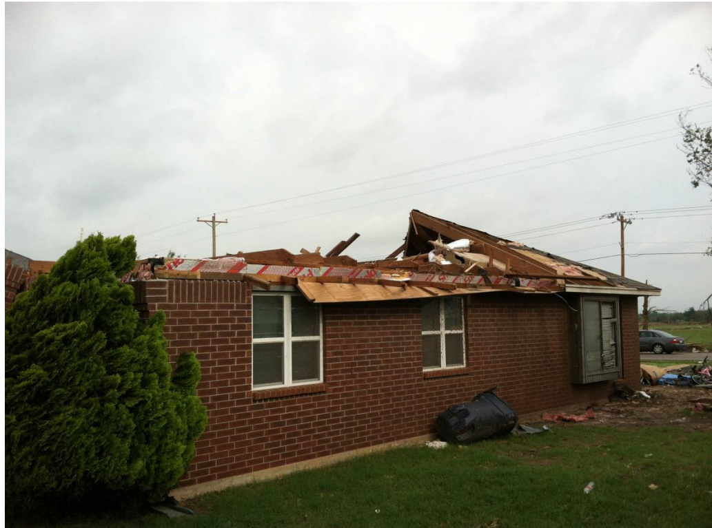
Figure 1-14 (Tornado Damage Assessment in the aftermath of the May 20th 2013 Moore Oklahoma Tornado, 2014)
