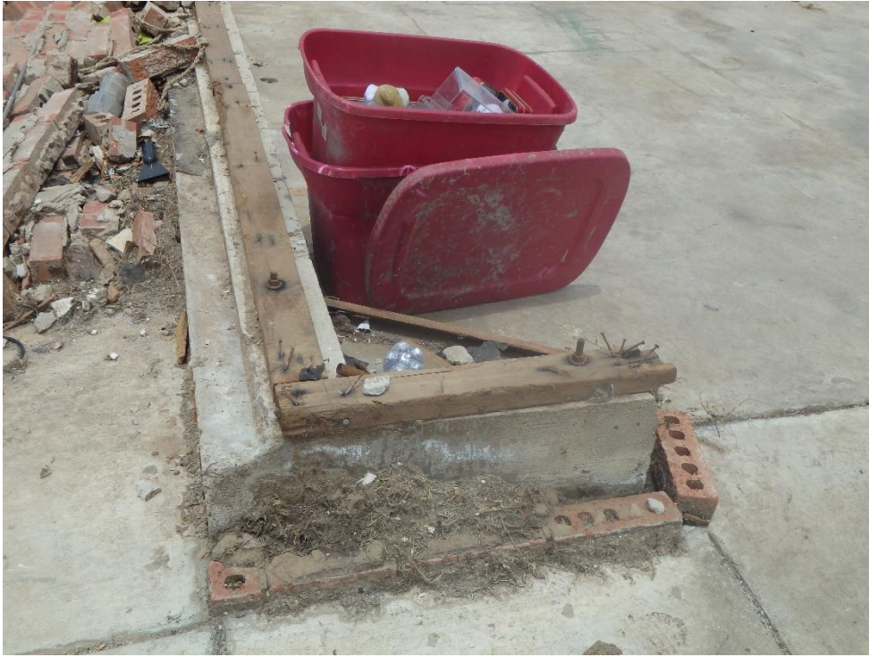
Figure 1-23 Undamaged Sill Plate, Failure of Sheathing to Sill Plate (Tornado Damage Assessment in the aftermath of the May 20th 2013 Moore Oklahoma Tornado, 2014)
