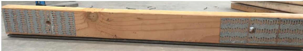
Figure 4-4 (b) Bottom Face of SAMPLE#2 Specimen. No Sign of Crack Or Any Damage Can Be Seen.
