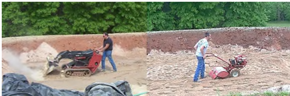
Figure 2- 3. On the left, a Dingo was used to evenly spread out the appropriate amount of fly ash for a filter layer lift. On the right, a roto-tiller was used to mix the soil amendment into the designated lift.
