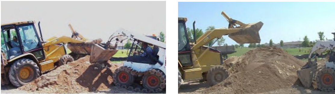
Figure 2- 2. Mixing fly ash into sand for filter layer using heavy machinery prior to placing into cells in 13 mm lifts.
