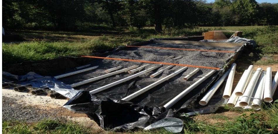
Figure 4.8. The subsurface drainage layer of a P removal structure was exposed prior to the addition of steel slag. The drainage layer used 10.16 cm diameter perforated PVC pipes.
