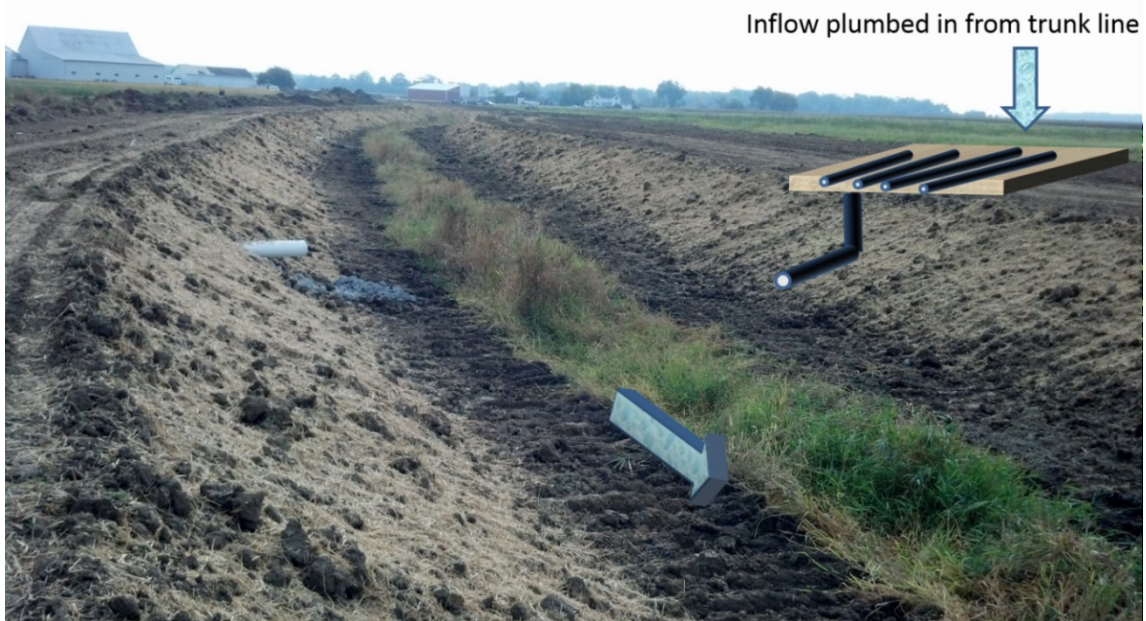
Figure 4.5. An example P removal structure design that uses a subsurface bed to treat a tile drain is shown.
