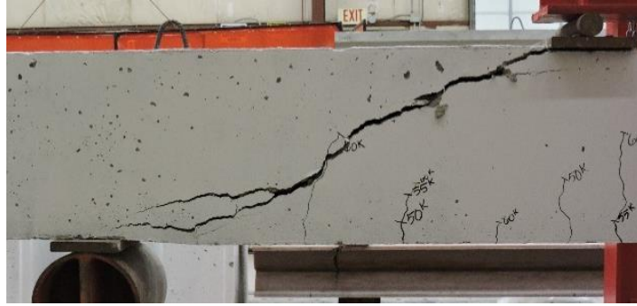
(a) K-C-1 Failure Crack
