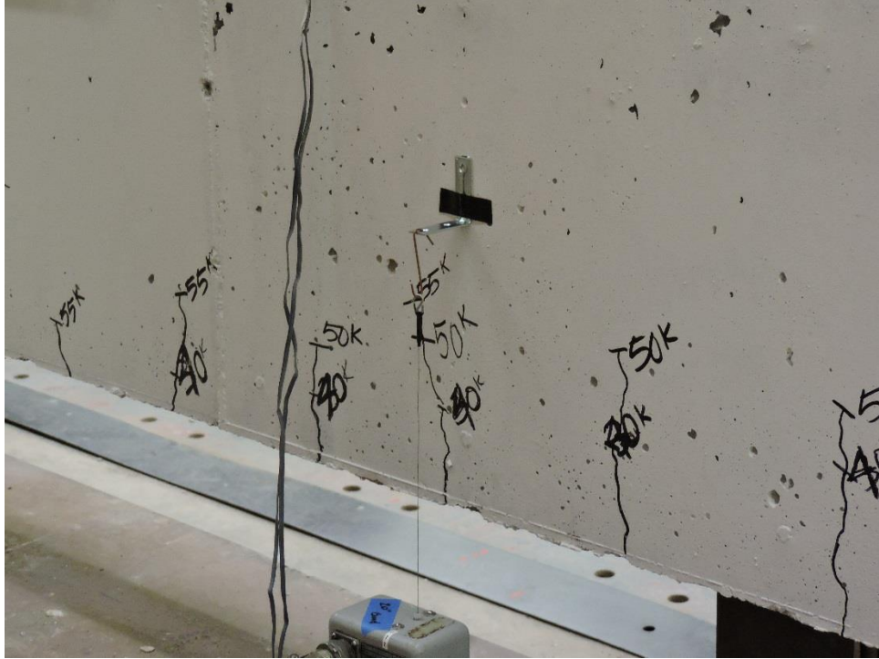
Figure A.3: K-C-1 Crack Propagation 55 kips
