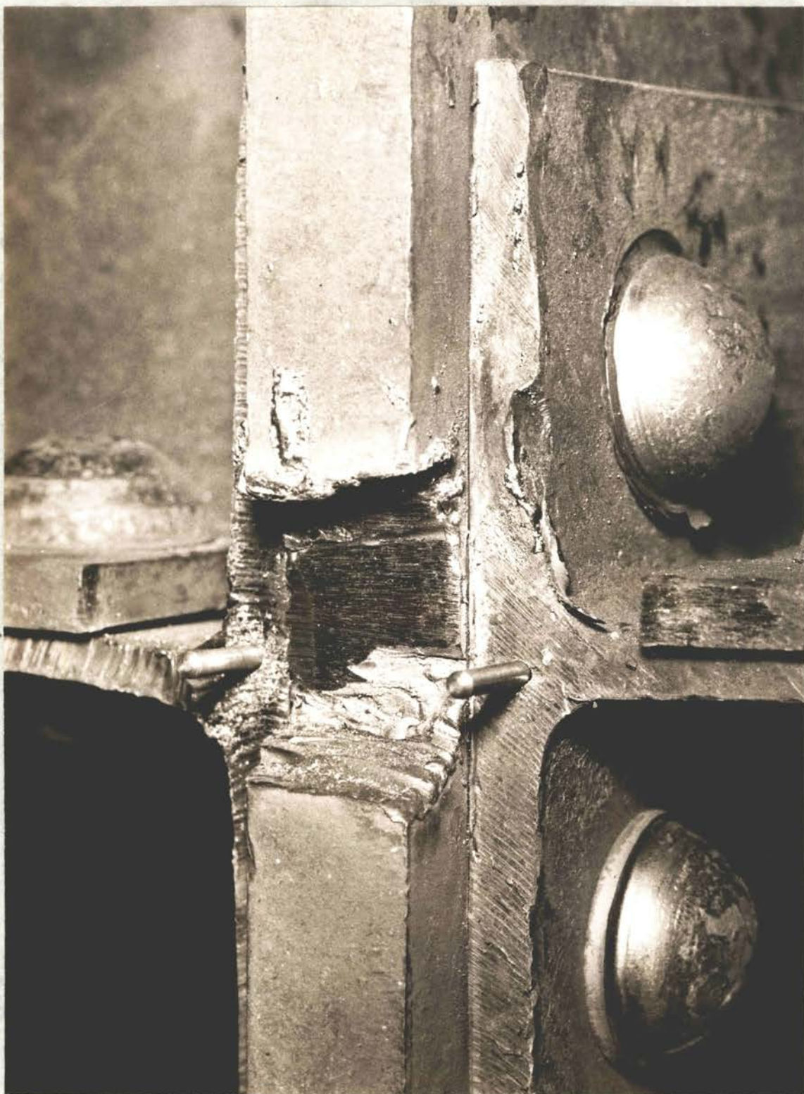
Fig. 11. Close up view of Tee flange for Specimen 1 showing slight crack between the plate and flange due to permanent set from a previous load.
