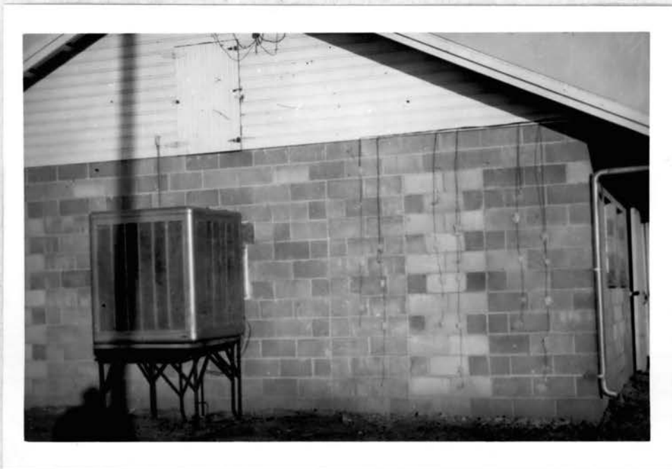
Fig. 5 - West Wall of Temperature-Controlled Shelter With Thermocouple Junctions Installed.
