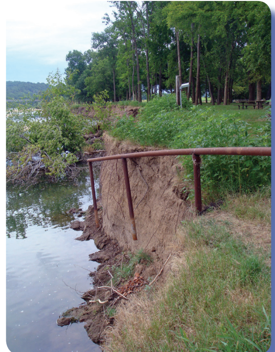
Picture above: Example of extreme bank erosion at the Illinois River
