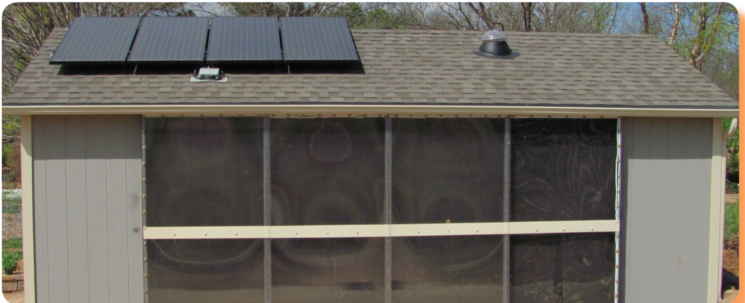
Picture above: Roof top solar photovoltaic panels at the OSU Botanical Gardens "Green Cottage".
