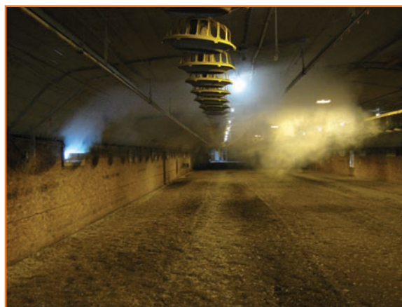
Figure 1: Photo of smoke test showing circulation pattern of air entering through building side vent.
