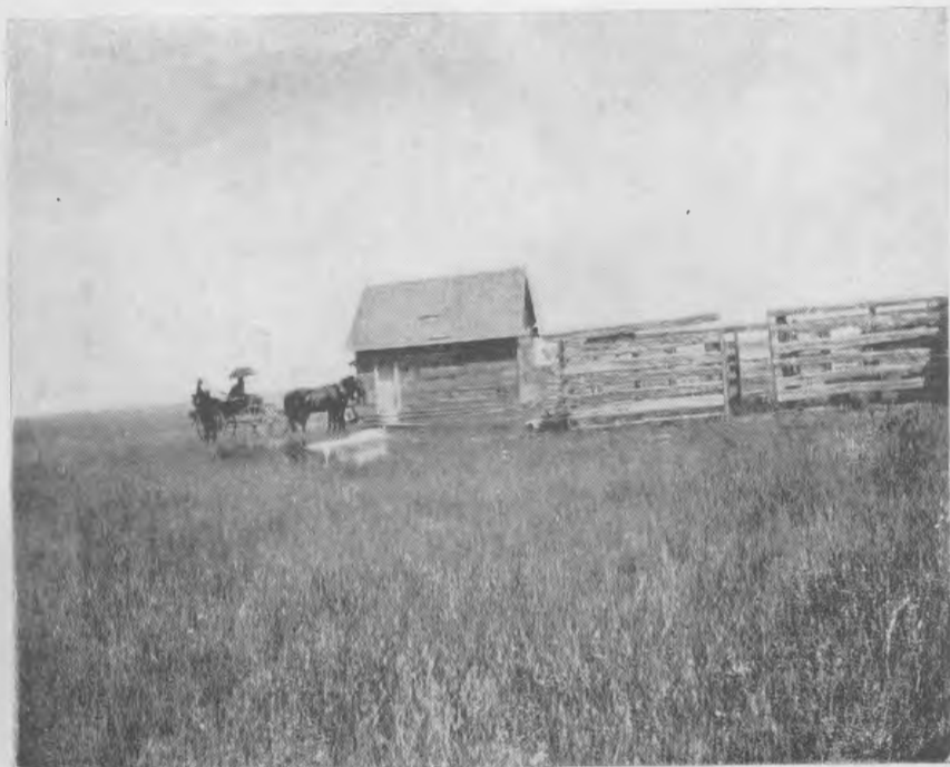
Thomas Tuttle's new house on his land. Pulling down the old log house to build the new.
