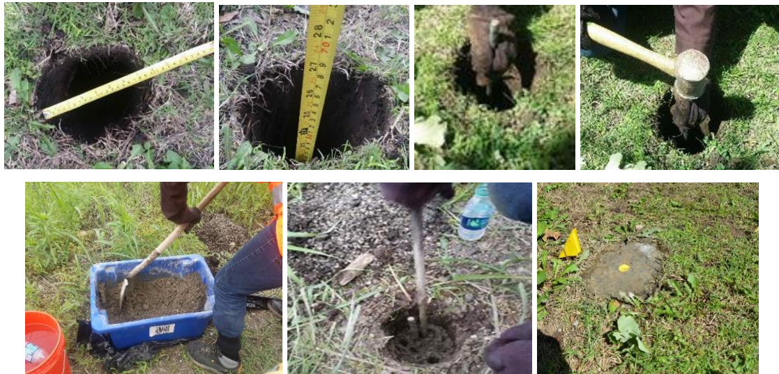
Figure 61: Different steps of installing survey benchmarks for Bridge No. 2 (Hatami et al. 2015)
