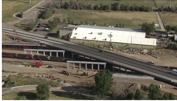
Figure 22: Bird view on the I-70 over Smith Road and Union Pacific Railroad Bridge construction site (Luber 2015)
