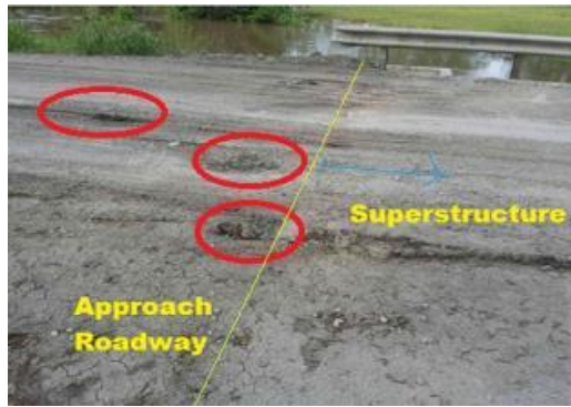
Figure 46: Potholes in the approach roadway of GRS-IBS Bridge No. 2 after the flooding event in May 2015
