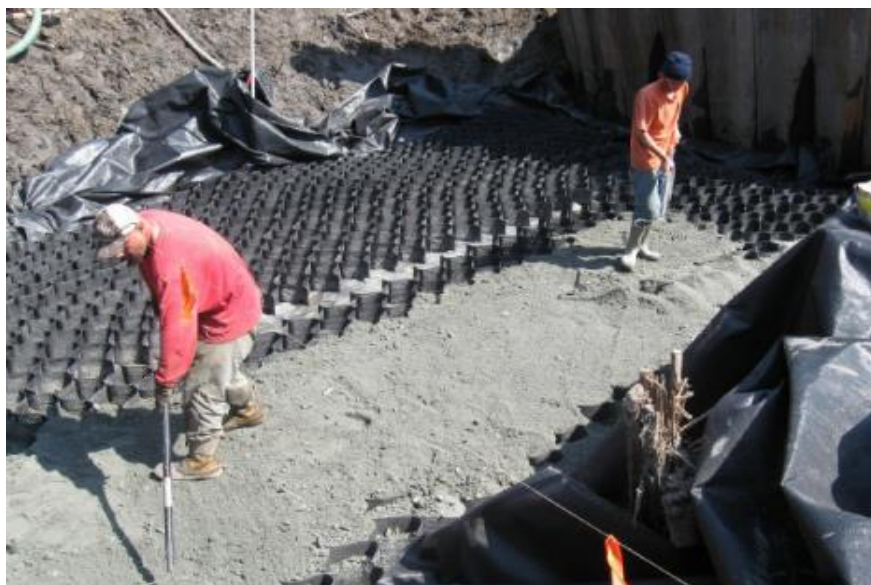
Figure 13: A cellular confinement system (CCS) with gravel infill was used for the Central Canal Bridge abutment in Hyde, North Carolina (Nguyen 2012).
