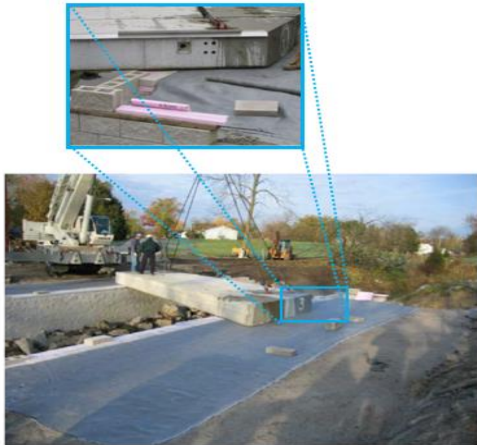
Figure 71: A geotextile is recommended in the FHWA guidelines (Adams et al. 2012) to be placed on the top of the GRS abutment before placing the beam seat
