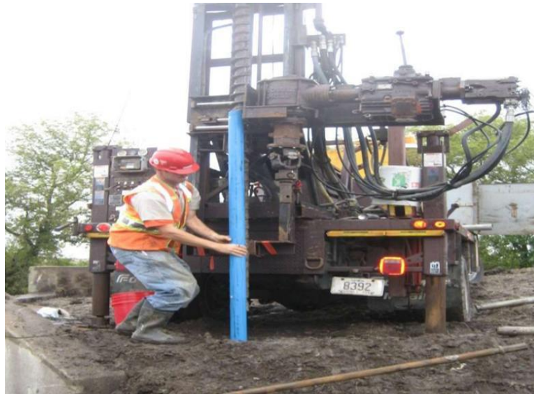
Figure 9: Installation of inclinometer for 250 th Street project in Iowa (Vennapusa et al. 2012)
