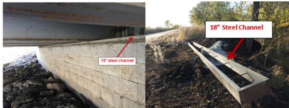
Figure 74: GRS-IBS Bridge No. 2 with an 18 in-wide concrete-filled steel channel as the bearing pad for the steel girders
