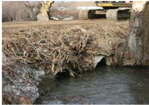
Figure 26: Damaged Culverts in Fergus County Road (Jenkins 2015)
