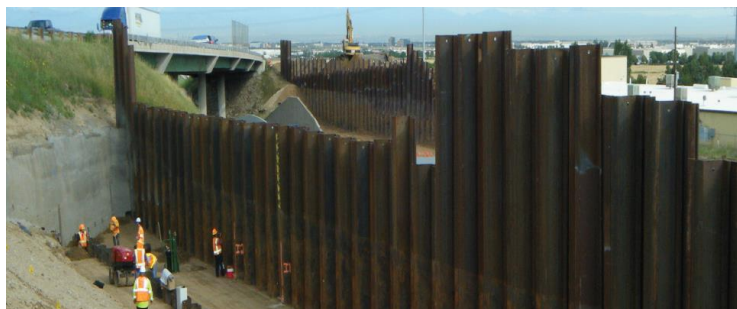
Figure 21: Sheet pile installation during I-70 over Smith Road and Union Pacific Railroad Bridge construction (Geocomp 2014)
