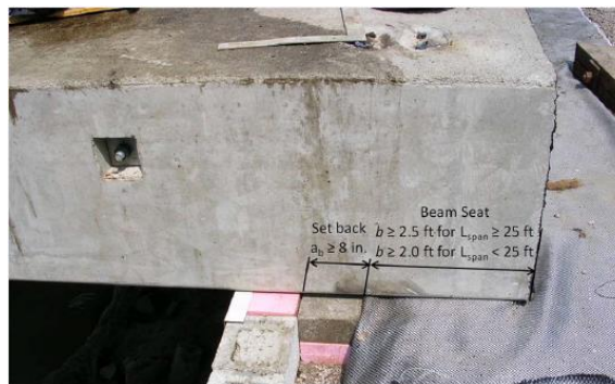
Figure 73: Setback for the beam seat as recommended by FHWA guidelines (Adams et al. 2012)
