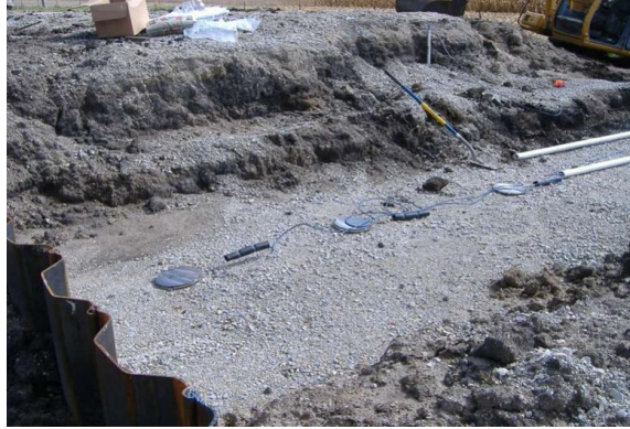
Figure 10: Installation of earth pressure cells for 250 th Street project in Iowa (Vennapusa et al. 2012)
