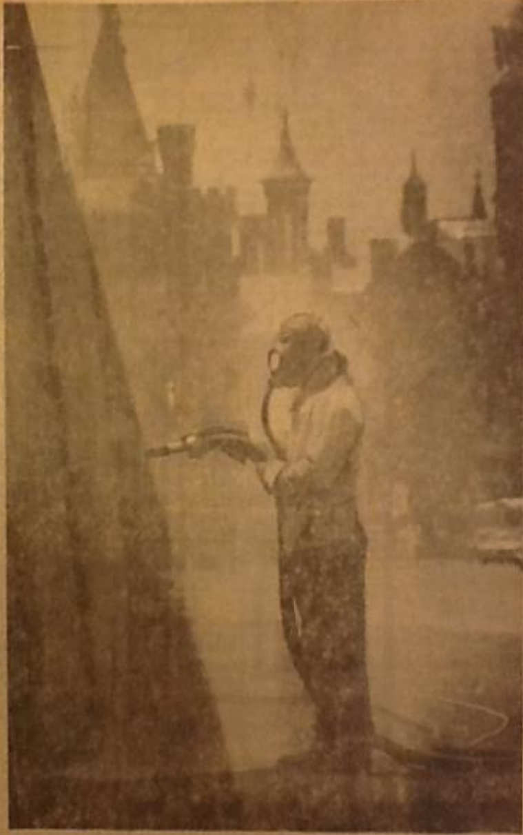
FUTURISTIC TOUCH — Looking like a space man, this worker sandblasts wall of the new Hirshhorn Museum of Modern Art, now under construction on the Mall, while “sculpture” of the Smithsonian Institution fronts gallery and looks to the background.
