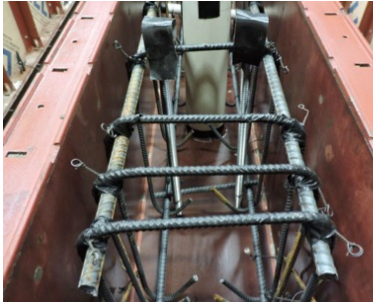
Figure 4.15 Stirrups Covered in Electrical Tape
