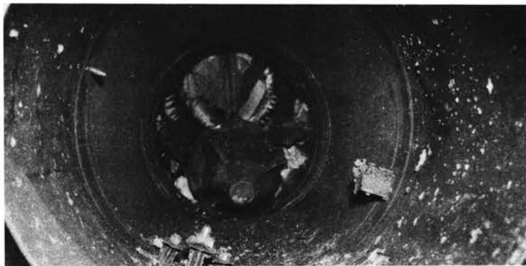
Damage is clearly visible through the tailpipe.
