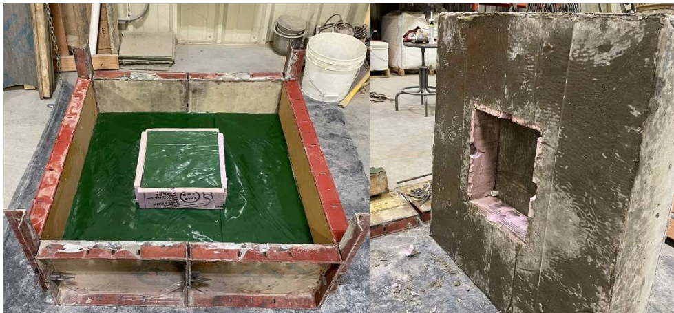
Figure 24 – Insert formwork before casting (left) and insert removed from bottom of slab (right)
