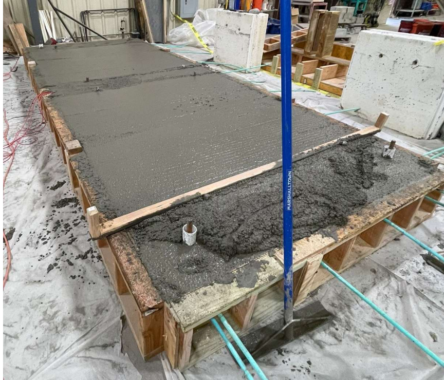
Figure 32 - Screeding and finishing the concrete to the approximate scaled slab elevation of 8 in.
