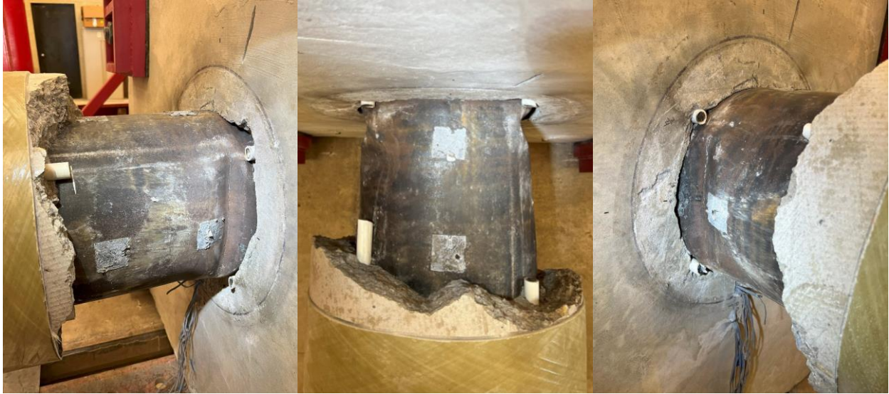
Figure 5-25: HS-SCC 2 Steel Tube West (l), Top (m), and East Side (r) Damage After Testing
