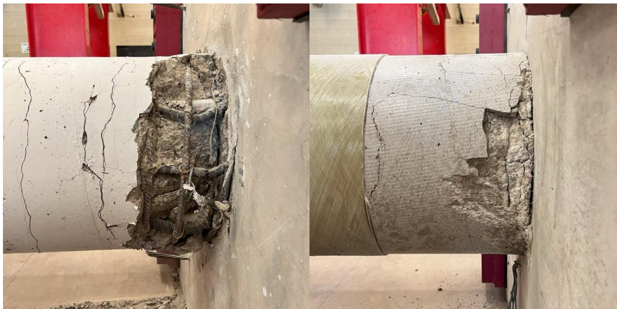
Figure 8-4: Comparing RC (l) and HS-SCC 2 (r) Concrete Core After Testing and Light Removal of Concrete
