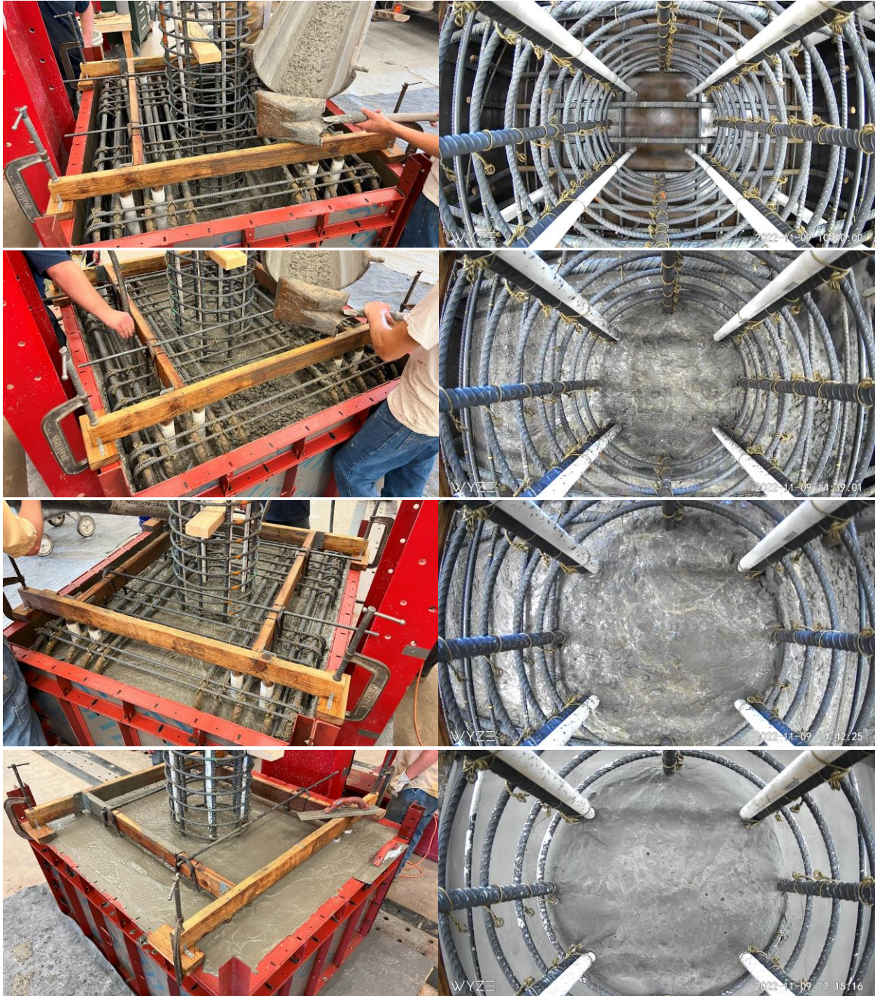
Figure 4-16: RC Column Base Casting at Various Heights, Column Base View (l) and Camera View (r)
