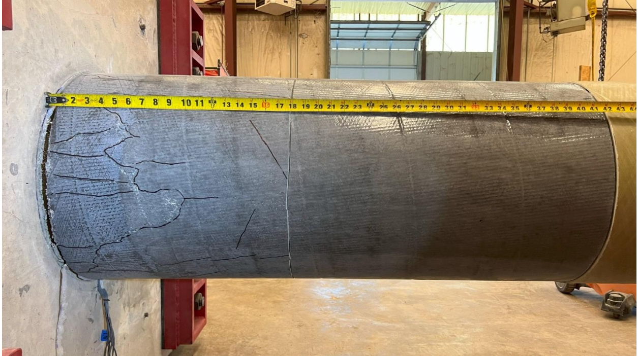
Figure 7-28: UHPC 2 Concrete Core East Side Cracking Along Column Height
