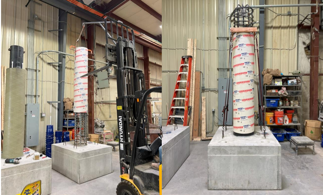
Figure 4-22: RC Column Form Placement and Preparation, Lowering the Form into Place (l) and Column Ready for Casting (r)
