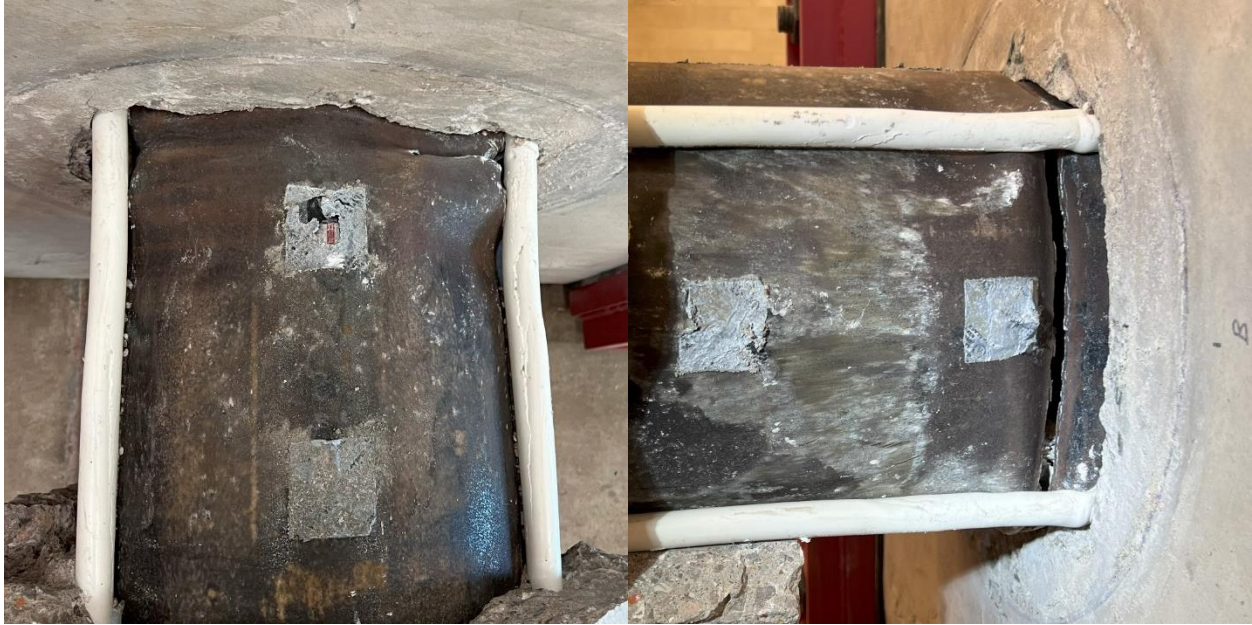
Figure 6-15: HS-SCC 1 Steel Tube Top (l) and West Side (r) Damage After Testing
