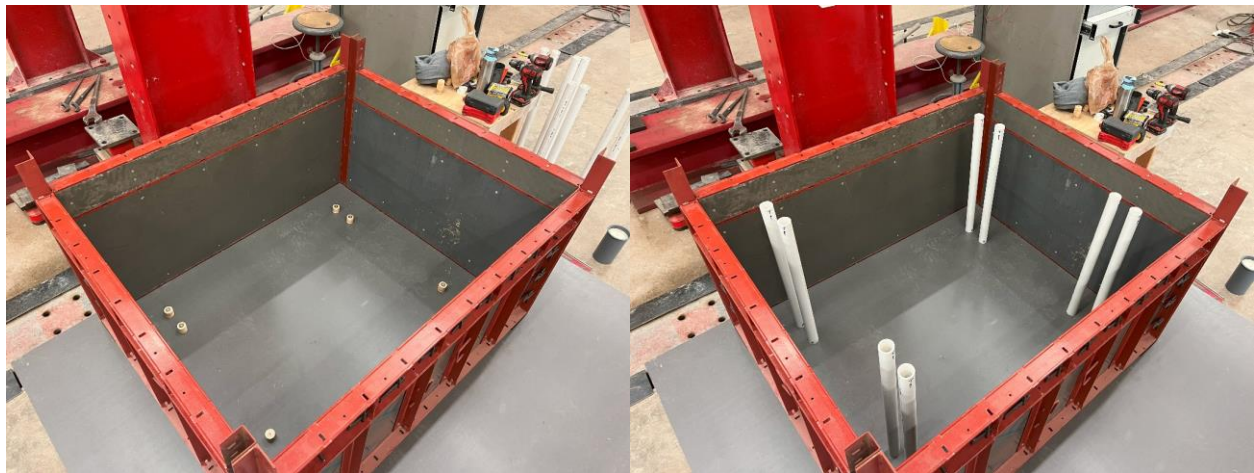
Figure 4-1: Column Base Formwork, Formwork Floor Dowels (l) and Base PVC Pipes (r)
