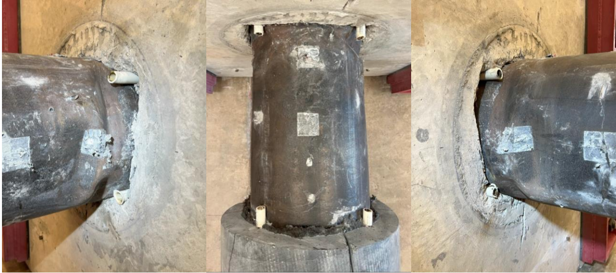
Figure 5-44: UHPC 2 Steel Tube West (l), Top (m), and East Side (r) Damage After Testing
