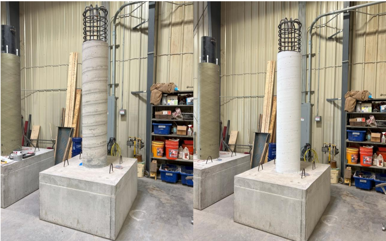
Figure 4-26: RC Column Specimen Before and After Painting
