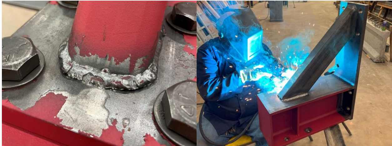
Figure 5-2: Loading System Fractured Weld and Reconstruction
