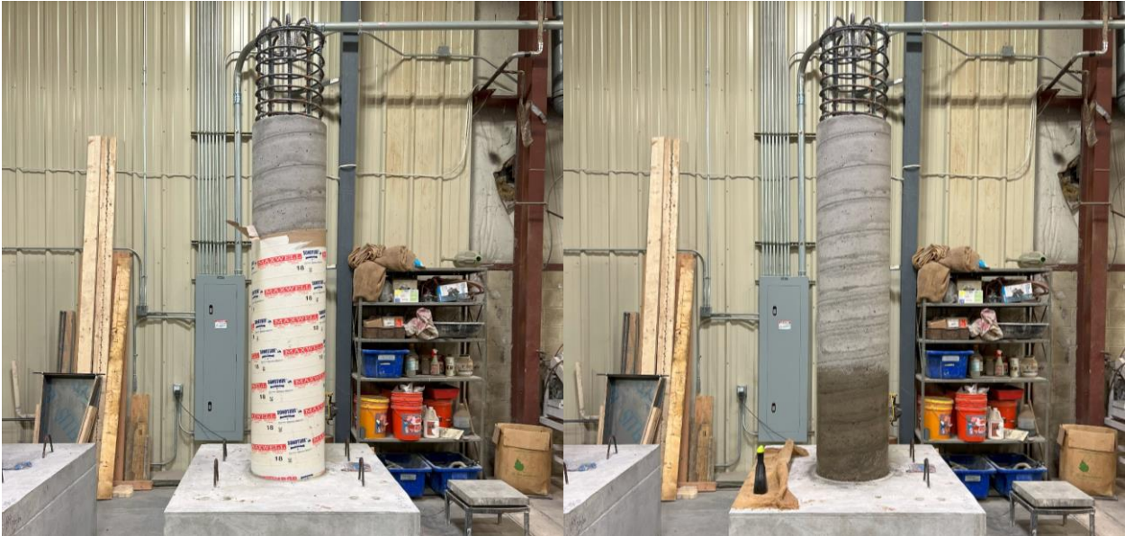
Figure 4-24: RC Column After Casting, Stripping the Form (l), Saturating Patch Area (r)
