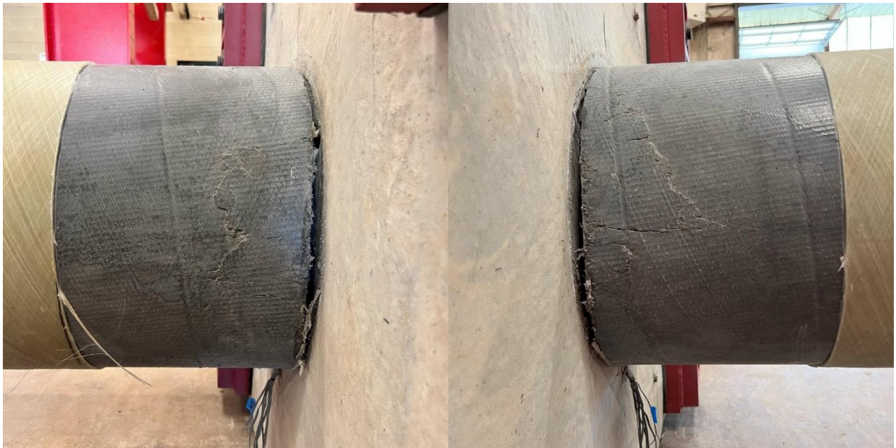
Figure 7-12: UHPC 1 Concrete Core West Side (l) and East Side (r) Damage After Testing
