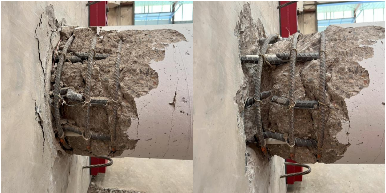
Figure 5-8: RC Column East Side After Testing (l) and Removal of Loose Concrete (r)
