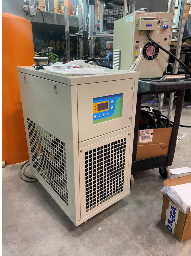
Figure III.10: Industrial Chiller Connected to Induction Heater
