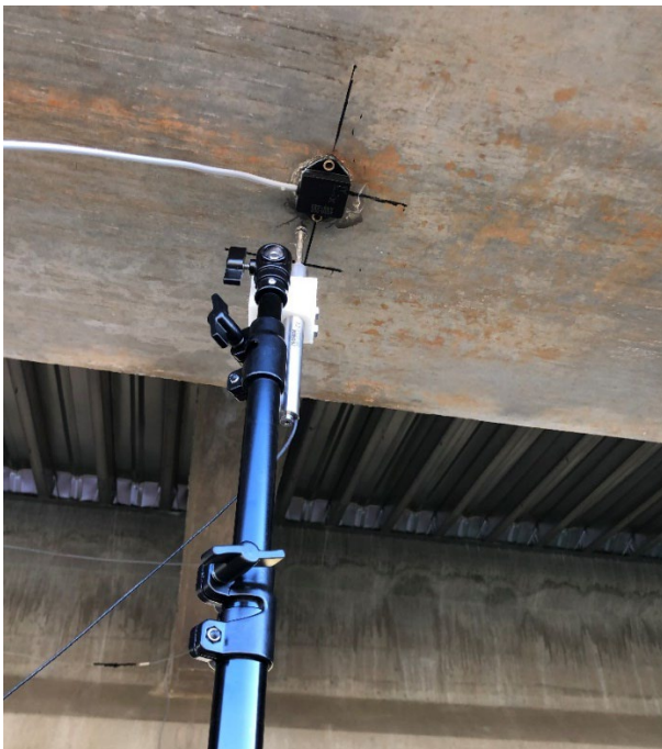
Figure 42: Instruments at midspan for SH 4 load test. Viewed are an LVDT and accelerometer.
