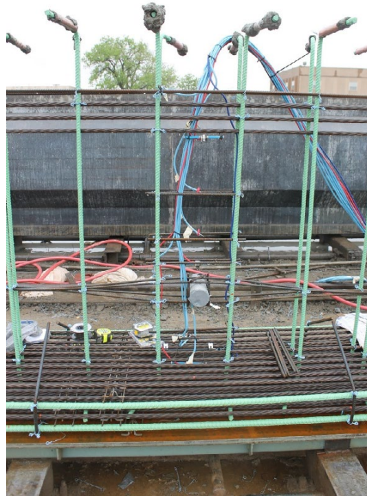
Figure 13: Instrumentation at midspan, Mark 27, Span 9. Four #7 reinforcing bars are placed in the corners of the bottom flange.
