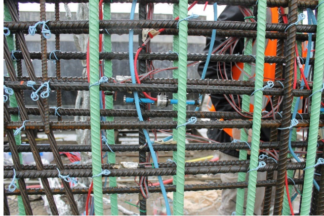
Figure 12: Vibrating Wire Gauge (blue) is located in the foreground at approximately C.G.S.
