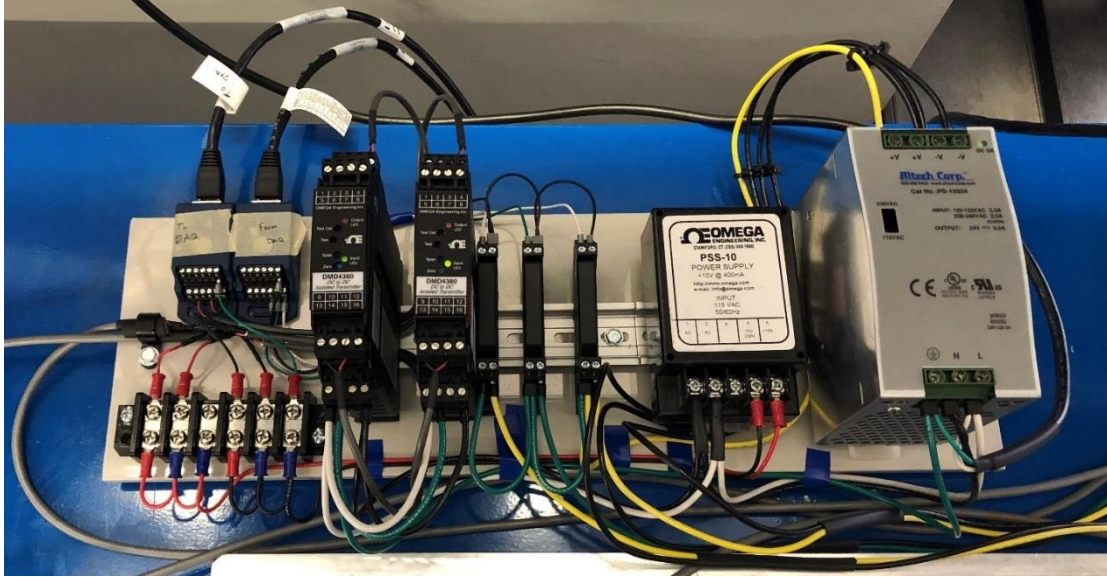
Figure 30: Bench wiring of power supplies, signal conditioners, and sensor leads
