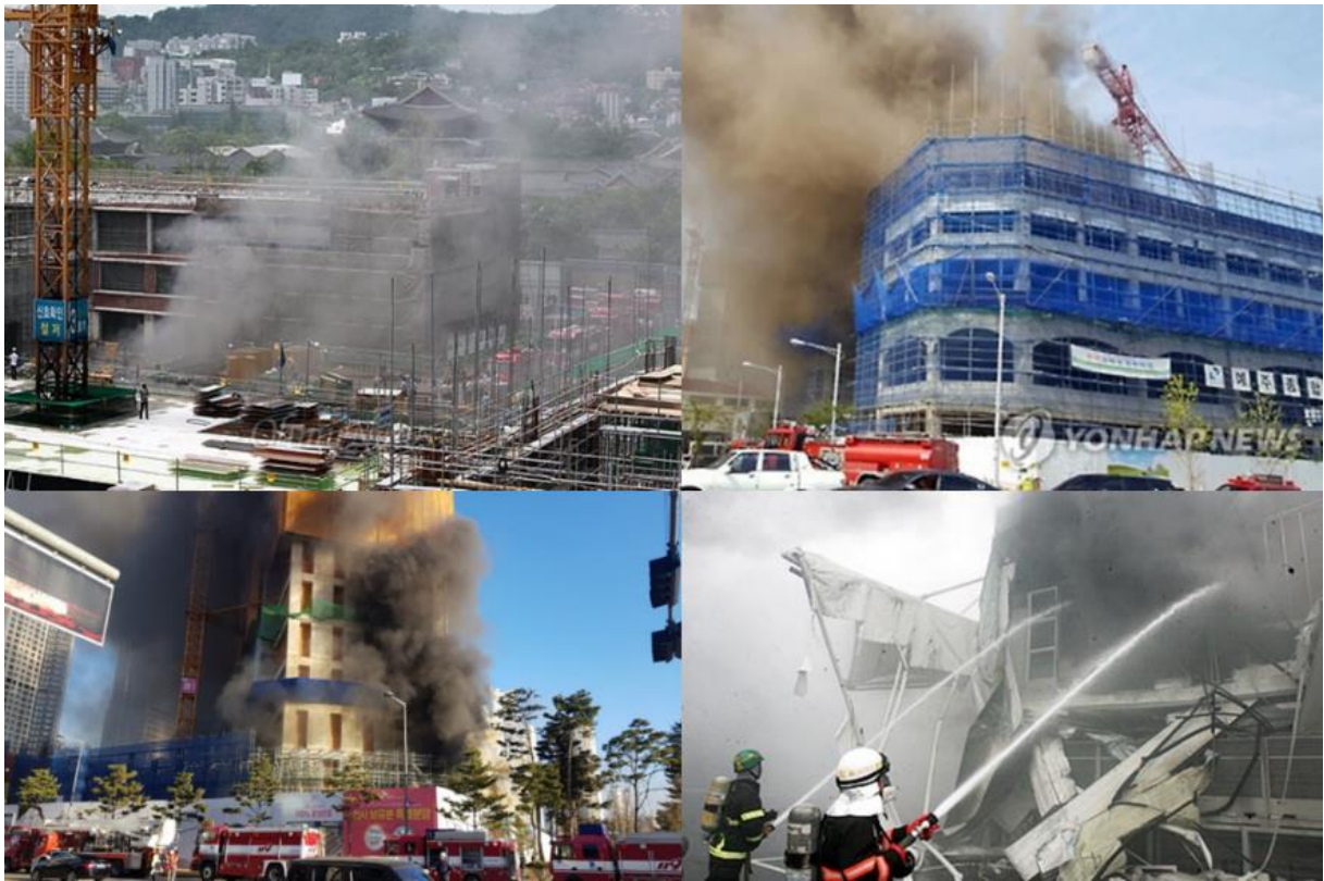
Figure 1-2 Examples of fire accident on construction site in South Korea
