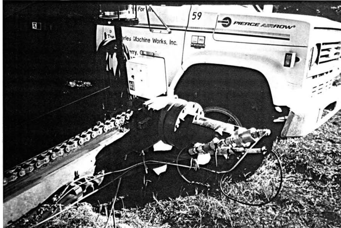
Figure 12: Position/velocity transducer mounted at back of boring unit. Note the pressure transducers at the inlet and outlet of the hydraulic thrust motor.
