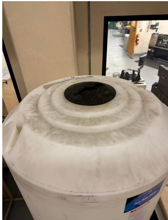
Image 2: Top of 300-Gallon Ace Roto-Mold Tank
