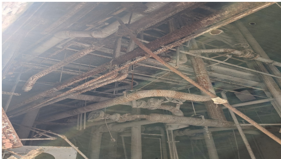
Figure 14 Asbestos from piping inside of the powerhouse during a site tour in October 2022. Source: Valerie Doornbos
