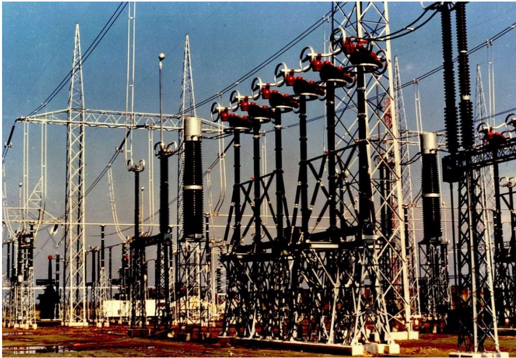
Figure 13 An open yard high voltage switch gearInvalid source specified.
