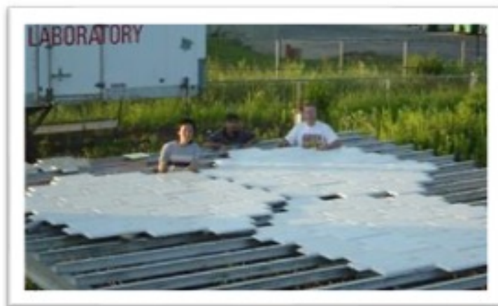
Figure 3.4: TEP array under construction in the field. Clutter fences, the transmit horn, and the trailer are visible in the background [70].
