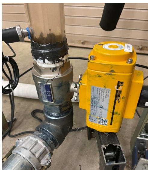
Figure 3-4: Quick closing valve at the bottom of the test section
