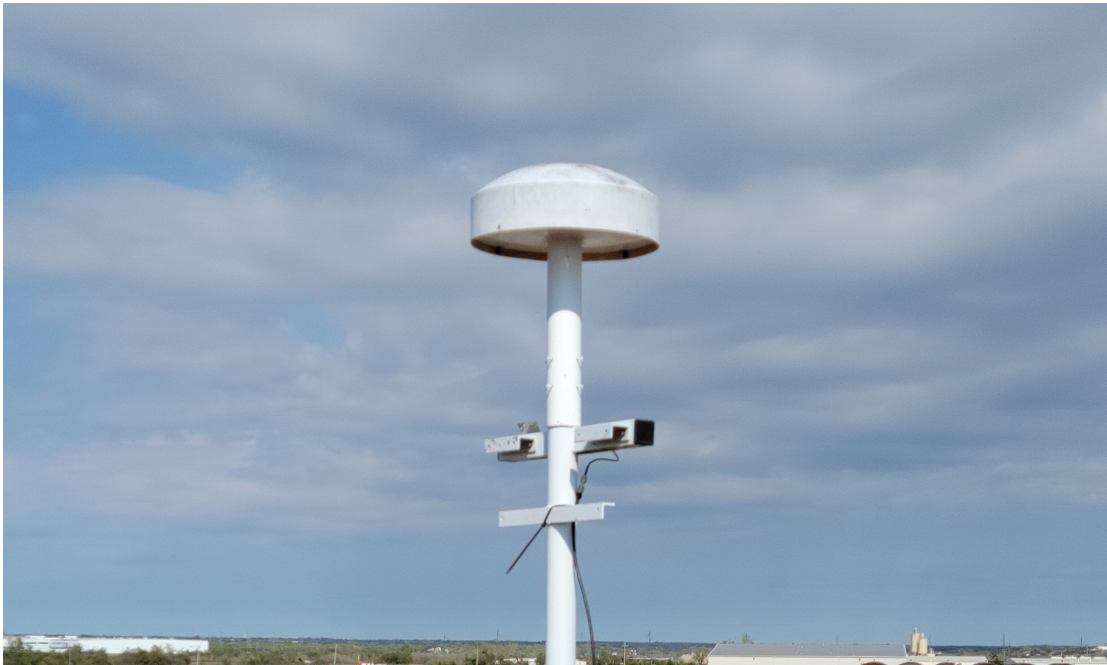
Figure 2.4. GPS Antenna: An image of the GPS-702-GG antenna installed on the roof of the LGF inside a multipath mitigating enclosure.
