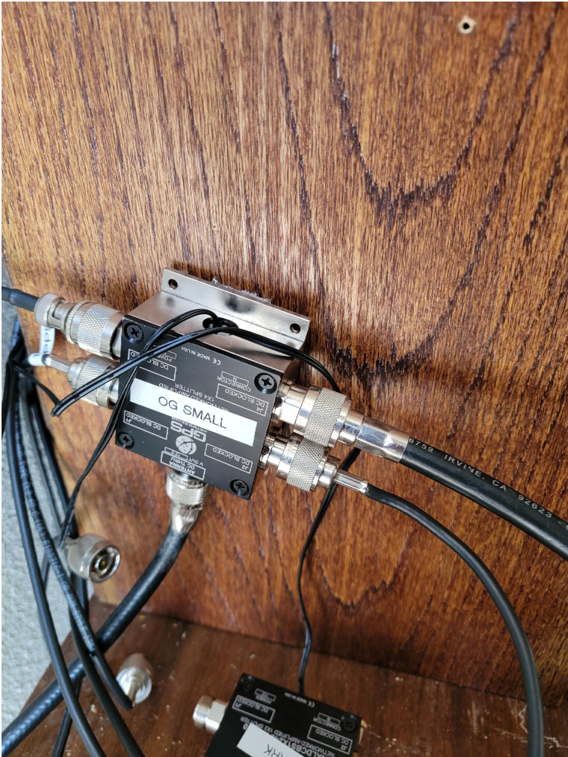
Figure C.5: Cables from the walls run directly to these GPS Networking active antenna splitters. In some instances, multiple 4x1 splitters are connected together to allow up to 7 different receivers to use the same antenna, as seen in the pseudorange testing in Chapter 4.
