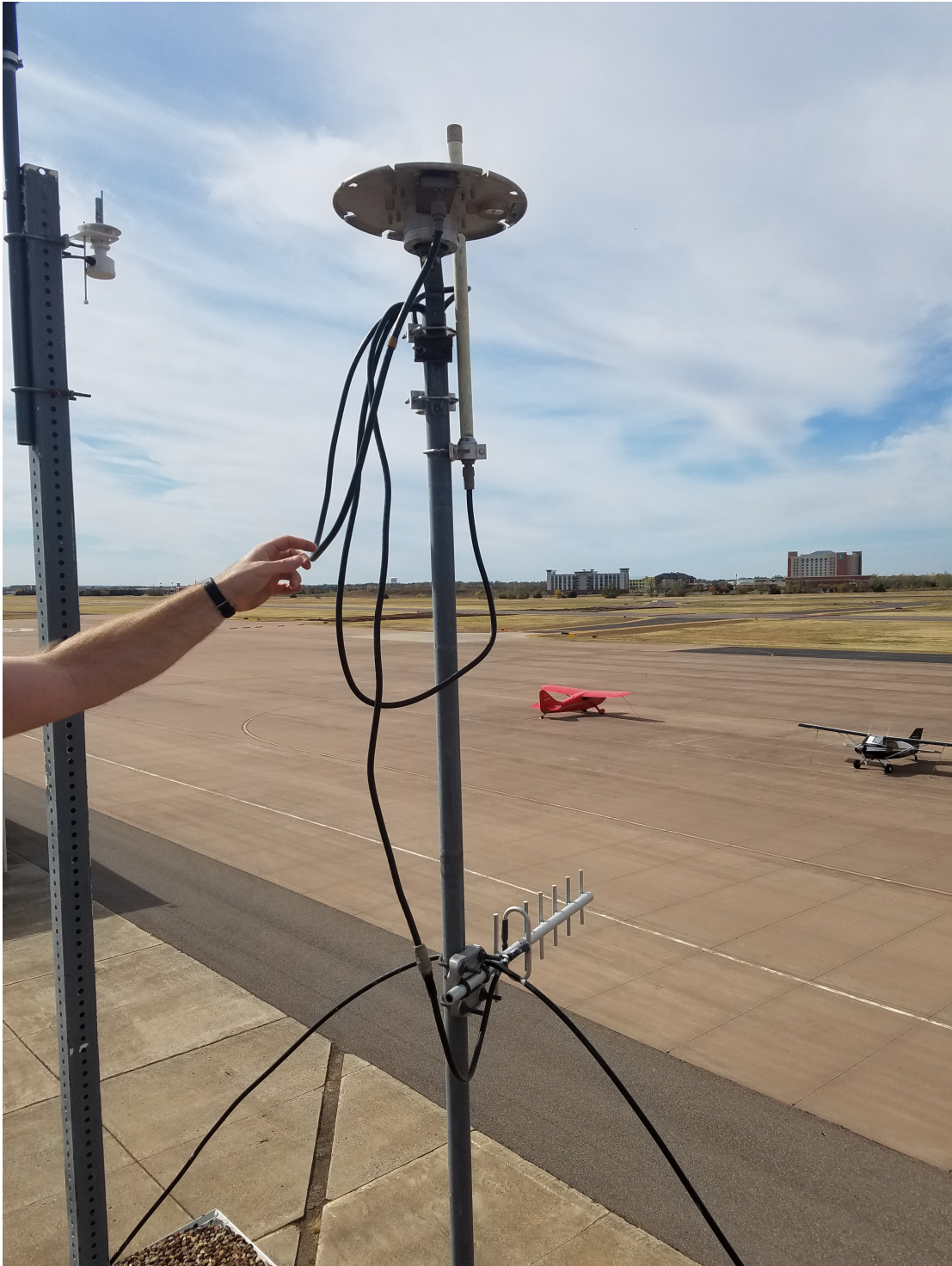
Figure C.2: The original OU GBAS local monitor antenna. This antenna is labeled “D” in Figure C.1.
