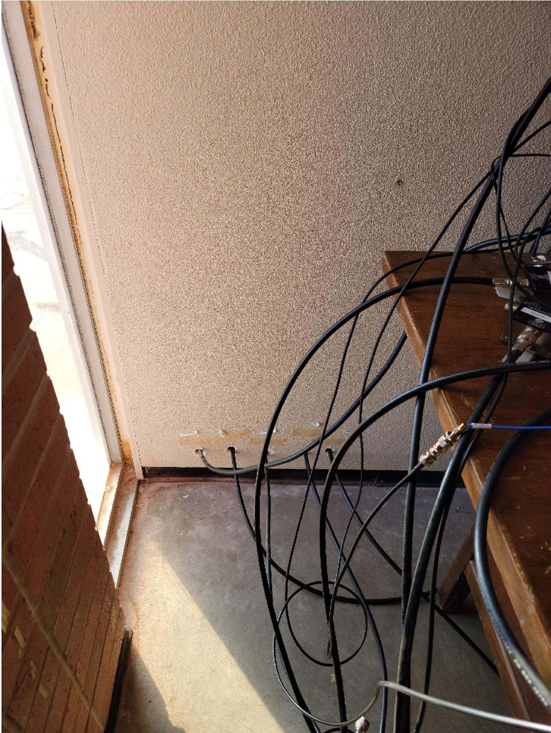
Figure C.4: Cables from the antennas located on the roof running into the GBAS room.
