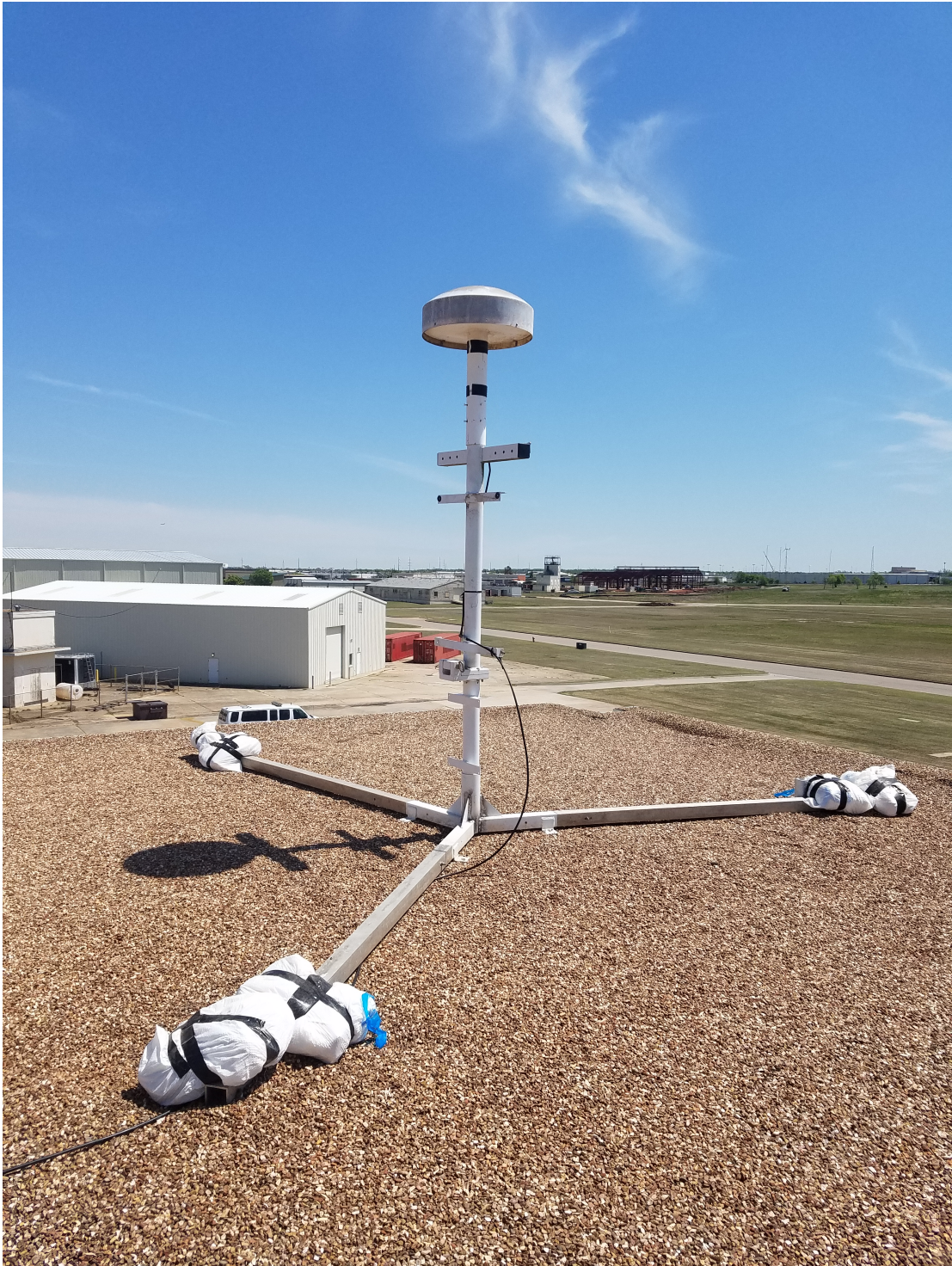
Figure C.3: The “Parking Lot Antenna” as labeled “A” in Figure C.1. Antennas labeled “B” and “C” are the same type of antenna.
