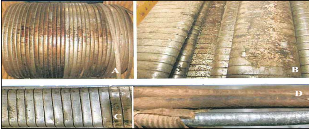
Figure 3-17: MLE Cable Dismantle Observations (Well #2), A) cable's external condition, B) cable armor's condition, C) a spot in the armor at 935' from MLE, D) opening in the cable armor, the lead insulation pressed.
