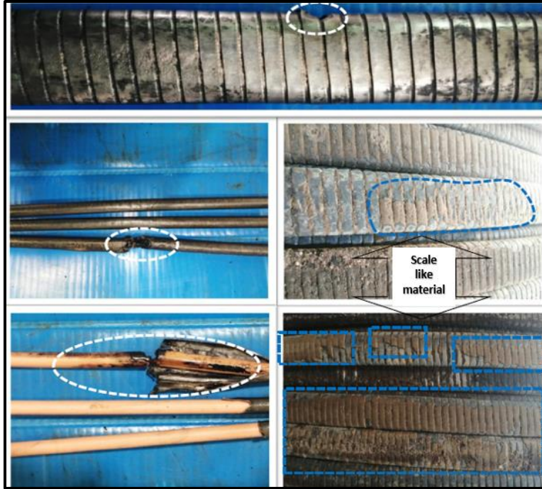
Figure 3-13: MLE Cable Dismantle Findings (Well #1)
