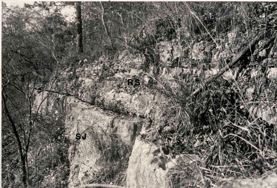
Figure 1. Reeds Spring (RS) limestone and chert beds converging against the upper bed of St. Joe (SJ) massive limestone; N. side of Spavinaw Creek, center of section 18, T. 22 N., R. 21 E.
