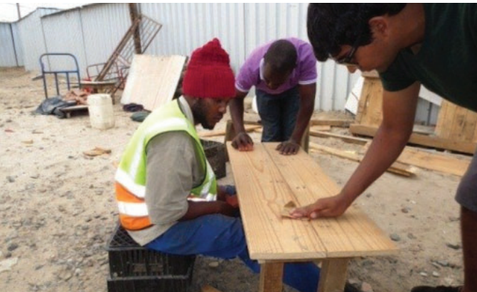
Reblocking, a participatory process that engages local residents in the reconfiguration of their shacks.
