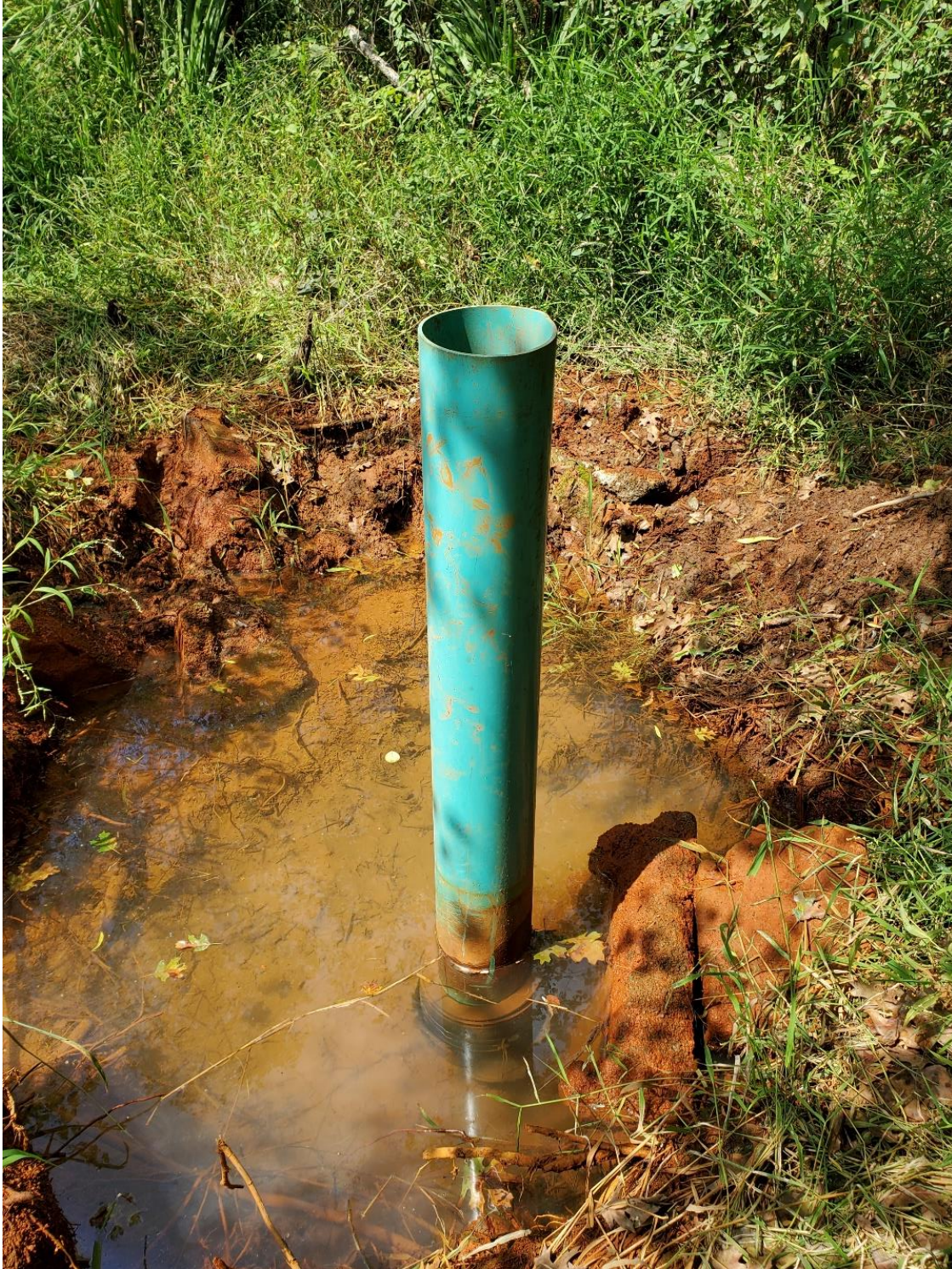
Figure 6A.2: Eight-inch riser installed on the S40 discharge. Photo taken September 4 th , 2021
