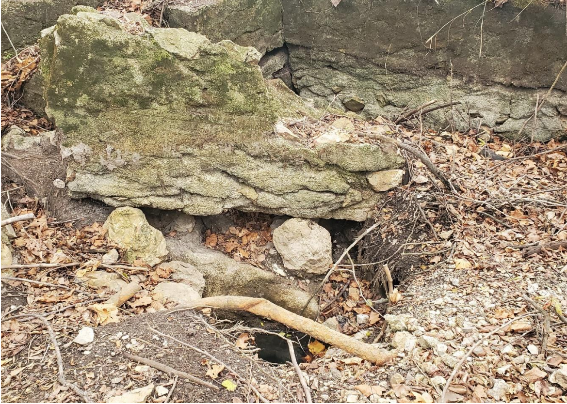
Figure 5B.10: Wesley Smith inflow location close-up of the partially open mine shaft, with large pieces of concrete lodged into portions of the opening. Photo taken in October 2020
