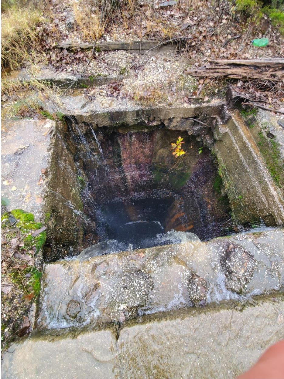
Figure 5B.16: Mid-Continent open mineshaft receiving runoff water during a rain event. Photo taken October 2019
