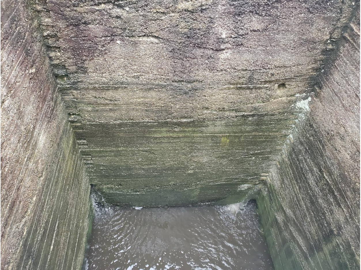
Figure 5B.21: Inside the John Hunt open mine shaft near Quapaw Creek, showing water entering through the concrete cracks on the corner of the shaft. Photo taken September 2019
