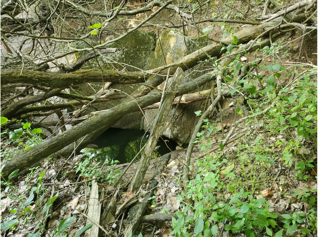
Figure 5B.8: Lytle 8 th St. inflow location during dry conditions, showing the rotated concrete cap and the mine pool water elevation under the cap. Photo taken in August 2021
