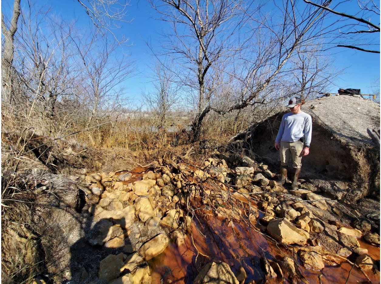
Figure 6B.5: Photo of the berm blowout at Flint Rock Discharge #1, with a student standing in the blown-out berm for size comparison. Photo taken February 2020
