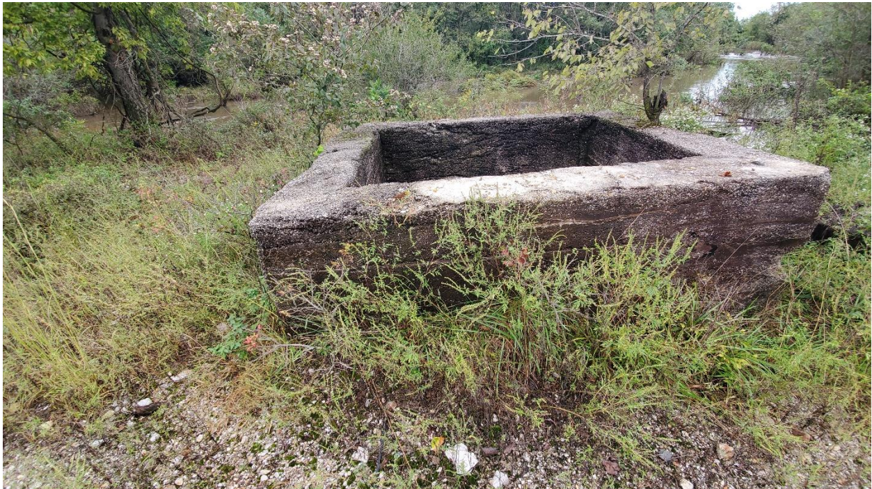
Figure 5B.20: John Hunt open mine shaft near Quapaw Creek. Photo taken September 2019
